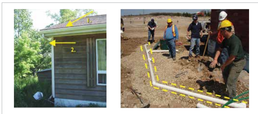
Figure I-1 Left 1. Gutter and 2. Downspout; Right Conveyance drainage piping for below-ground rainwater storage tank (prior to burial)
