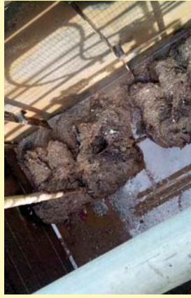
RAGS CLOGGING TANK
