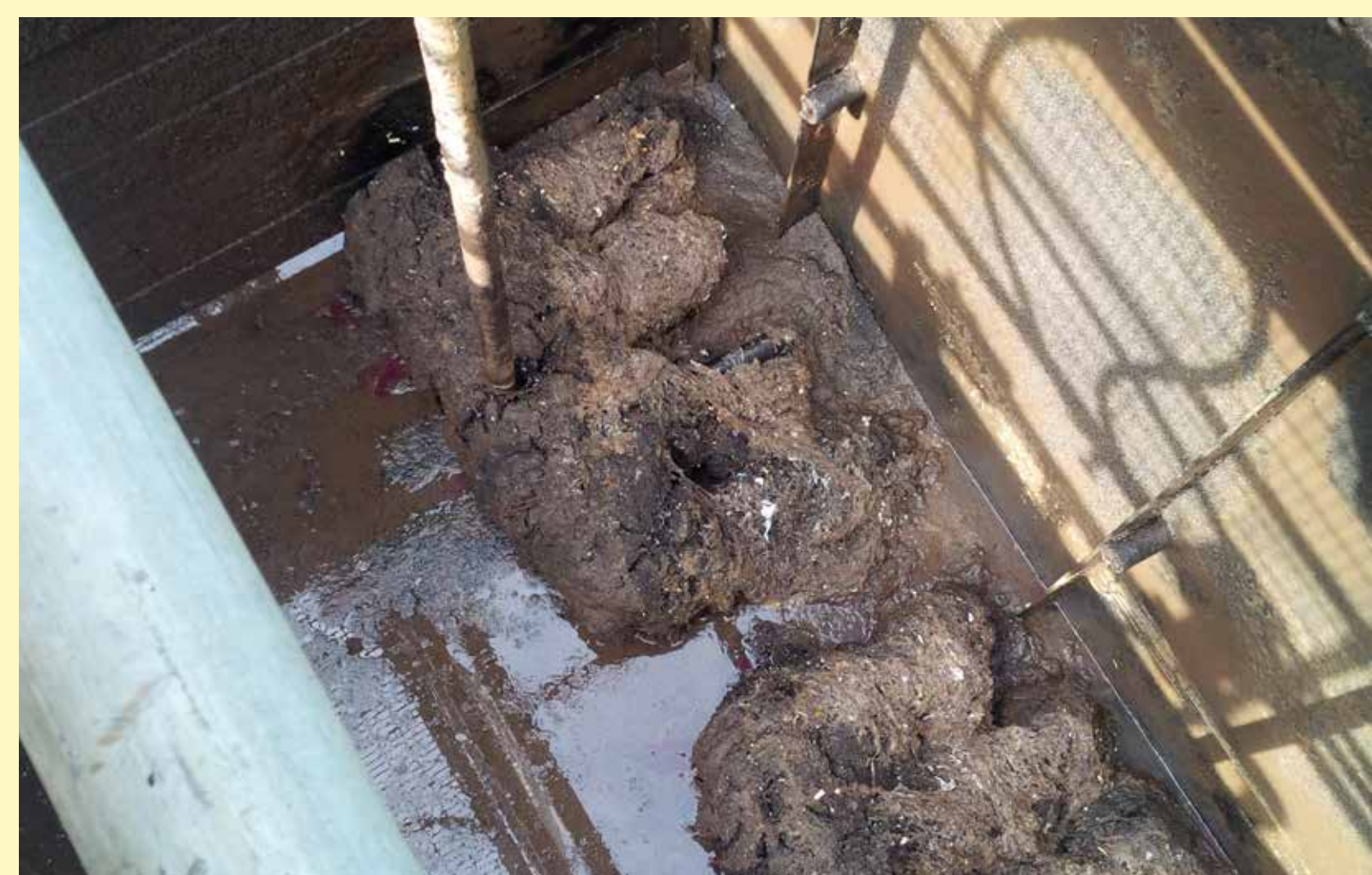
RAGS CLOGGING TANK
