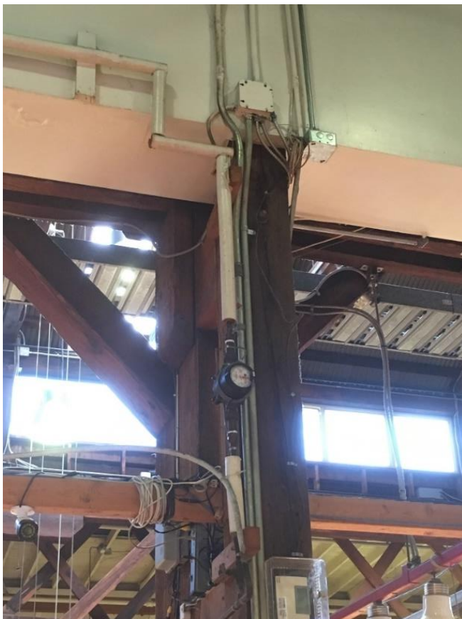
Figure 5. A water sub-meter near the ceiling, which measures the water usage of a produce store at the Public Market.
