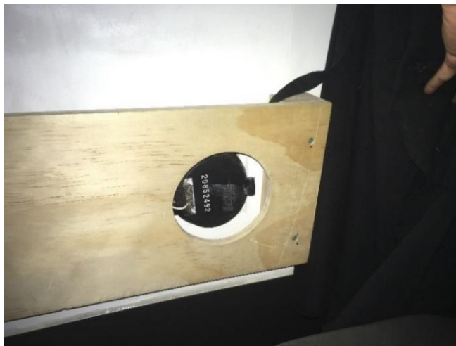
Figure 16. A water sub-meter, protected by a wooden case, installed in a bookkeeping space of a coffee shop.
