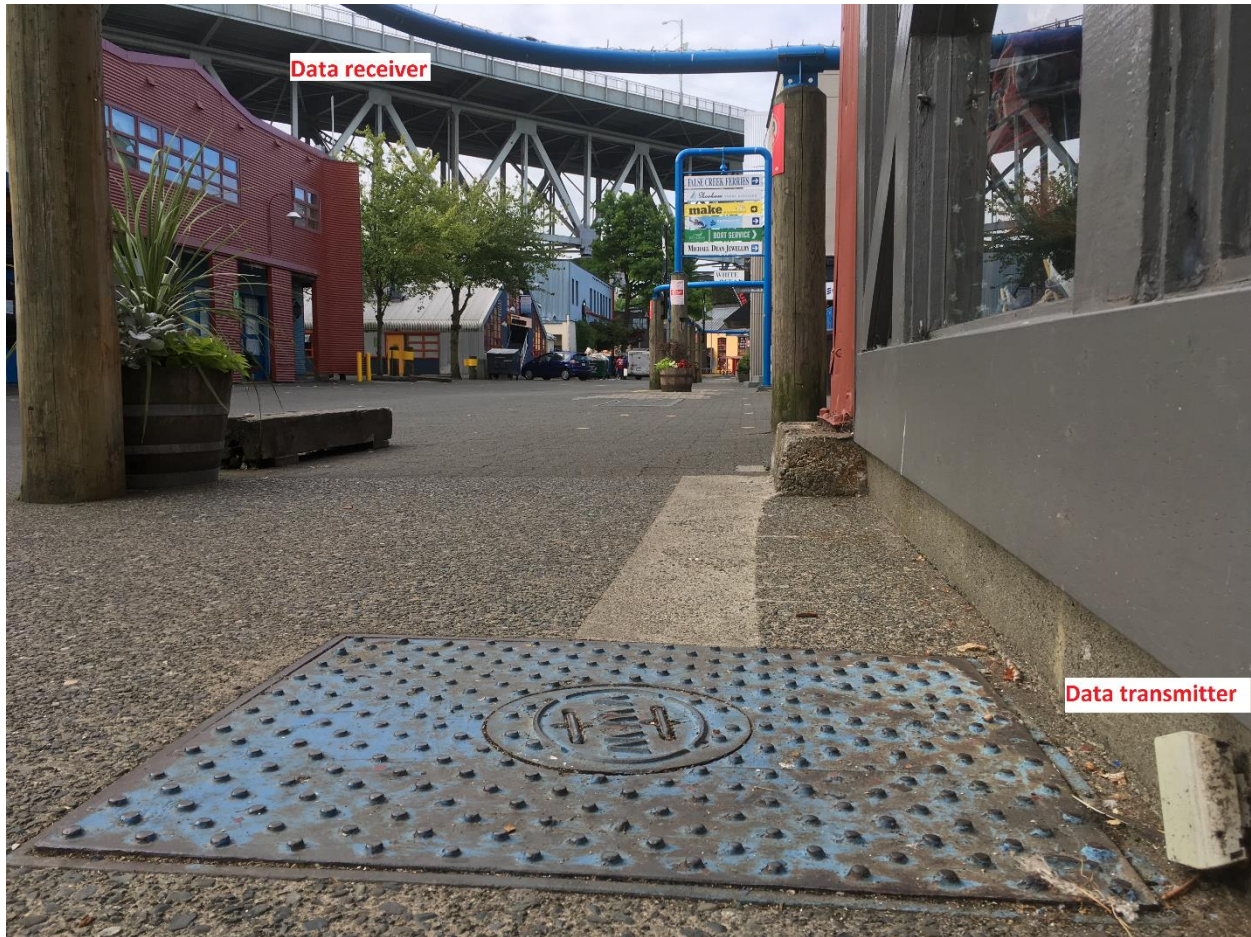
Figure 12. A GWF M-bus system outside a building on Granville Island
