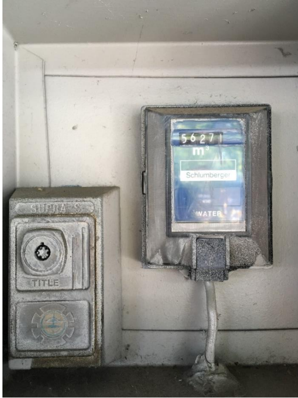
Figure 11. A manual reading water meter that measures the water use of a bakery on Granville Island.
