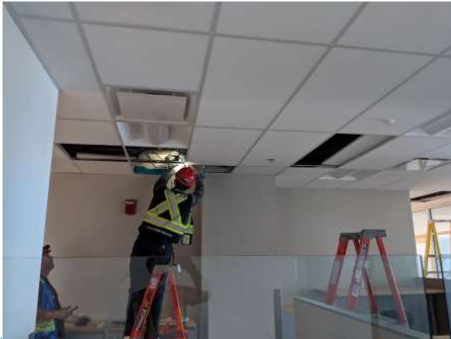
Figure 3– McLoughlin Point Wastewater Treatment Plant- Lighting controls installation in general office level 2.
