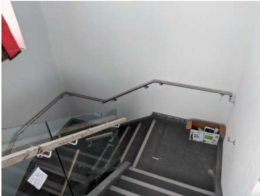
Figure 5- McLoughlin Point Wastewater Treatment Plant- Handrail installed in Operations & Maintenance main entrance stairwell.
