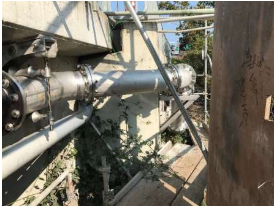
Figure 16–Residual Solids Pump Stations–Admirals Bridge additional pipe support bracket installed.
