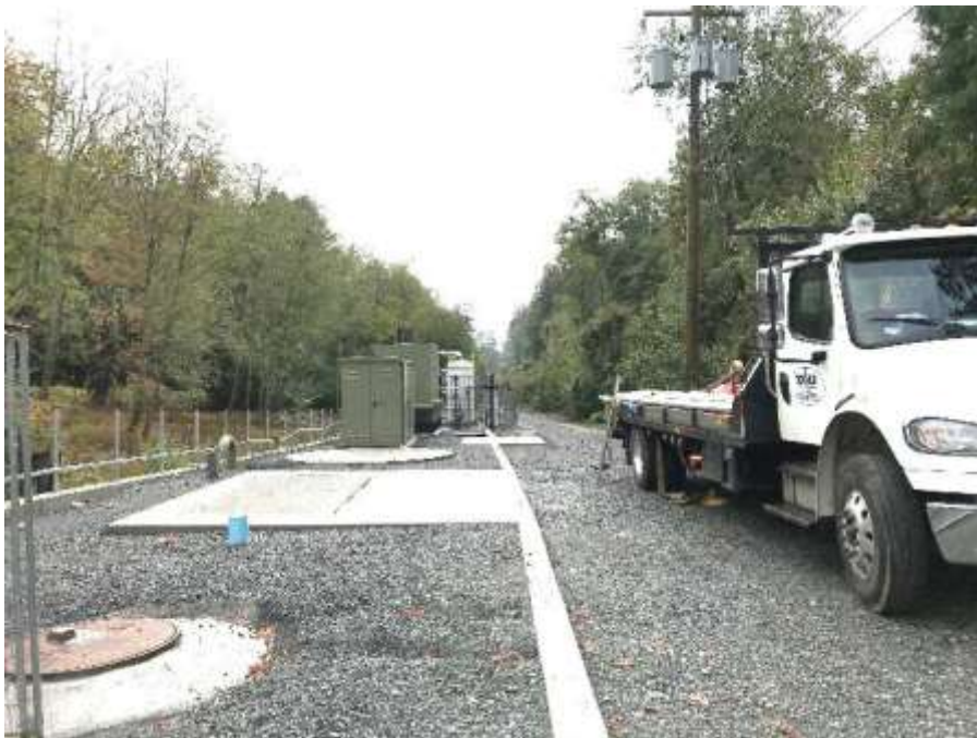
Figure 17 –Residual Solids Pump Stations – Pump Station 2- Tower Fence on-site installing fence on the retaining wall.
