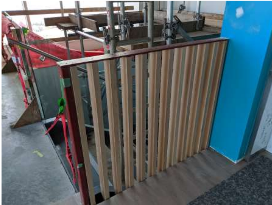
Figure 2– McLoughlin Point Wastewater Treatment Plant – Railing installation in Operations & Maintenance building main entrance stairway.
