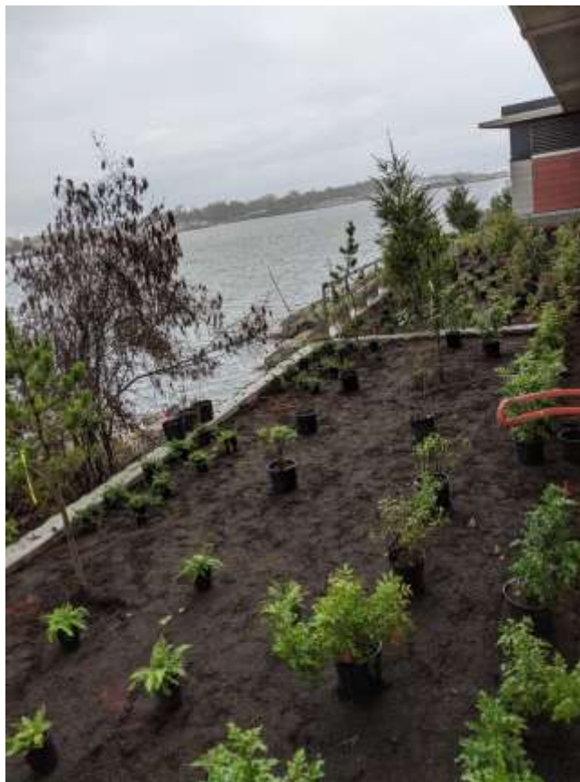
Figure 4– McLoughlin Point Wastewater Treatment Plant- Planting shrubs in planter next to Operations & Maintenance building workshops.
