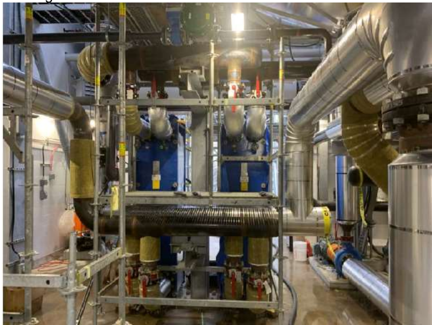
Figure 6- Residuals Treatment Facility- Pipe insulation being installed on Dryer building process piping.
