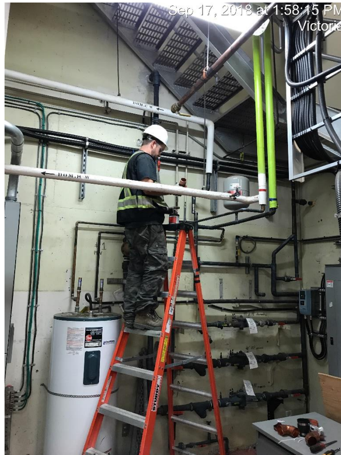
Figure 16 – Macaulay Point Pump Station: Installing temporary water service tie-in to existing pump station.
