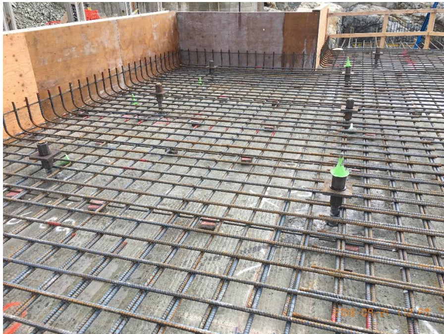
Figure 8 - McLoughlin Point Wastewater Treatment Plant: Installing anchor bolts and rebar for biological aerated filter (BAF) slab.
