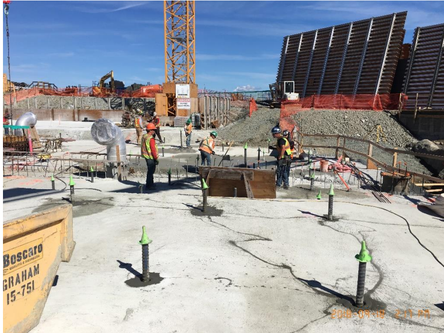
Figure 5 - McLoughlin Point Wastewater Treatment Plant: Grouting in anchor bolts for biological aerated filter (BAF) slab.
