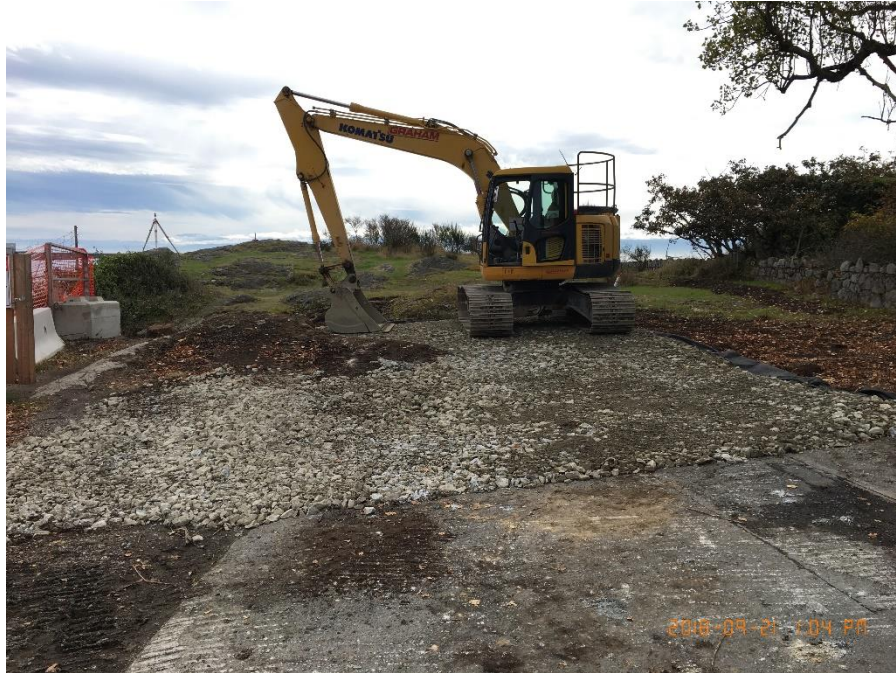
Figure 7 - McLoughlin Point Wastewater Treatment Plant: Preparing crane pad for hoisting the Micro Tunnel Boring Machine (MTBM).
