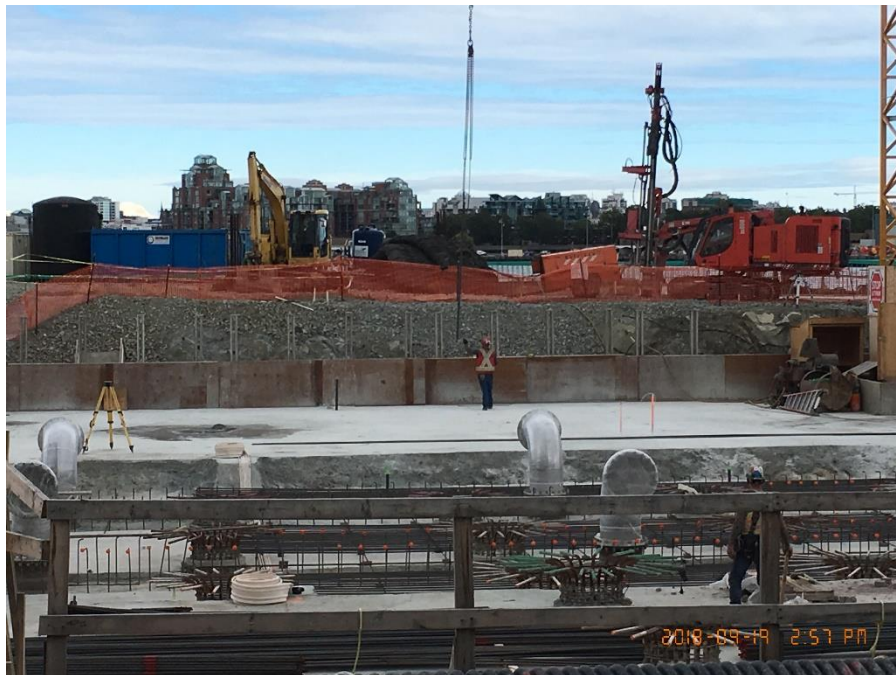
Figure 6 - McLoughlin Point Wastewater Treatment Plant: Installing biological aerated filter (BAF) slab formwork.
