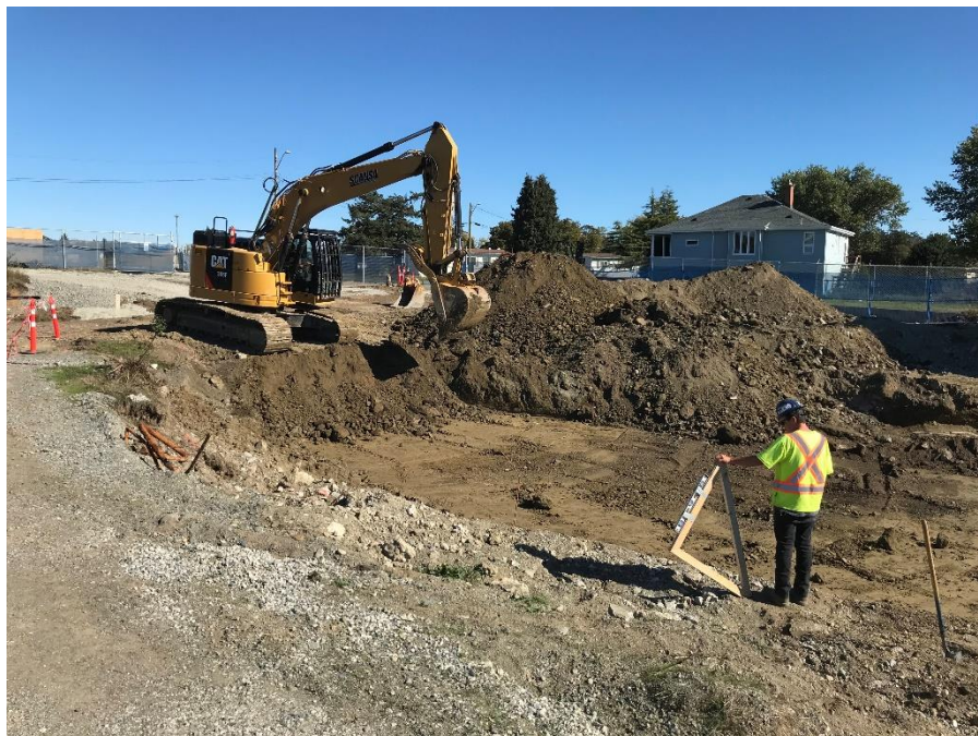
Figure 15 – Macaulay Point Pump Station: Commenced excavation of pump station footprint to bedrock.
