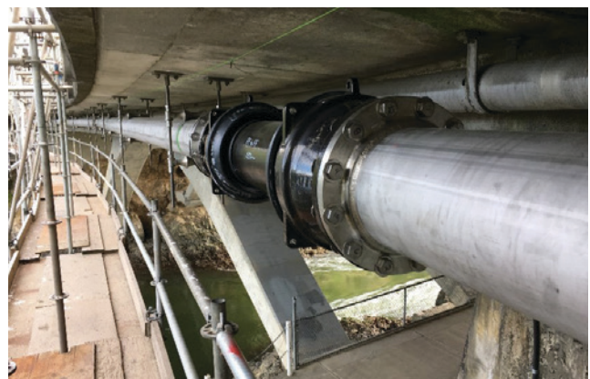
The pipe has been installed under the Gorge Bridge on Tillicum Road.
