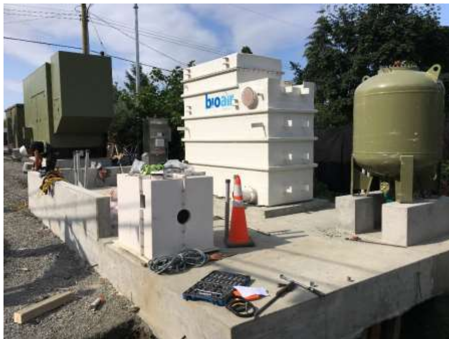
Figure 19 –Residual Solids Pump Stations – Pump Station #1.
