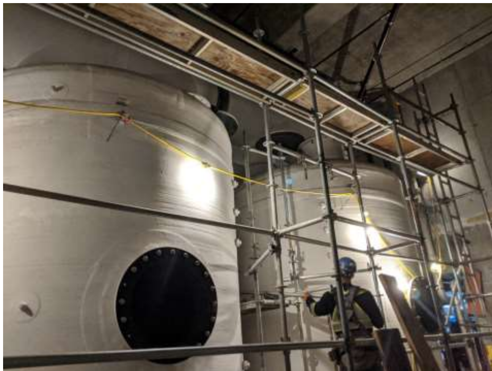
Figure 3- McLoughlin Point Wastewater Treatment Plant- Dirty Backwash Room, primary odour control carbon filter preparing to load media.
