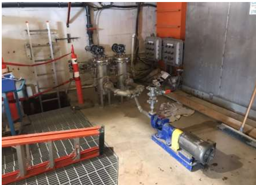
Figure 10–Clover Point Pump Station- Reclaim water system installed in the screening room.
