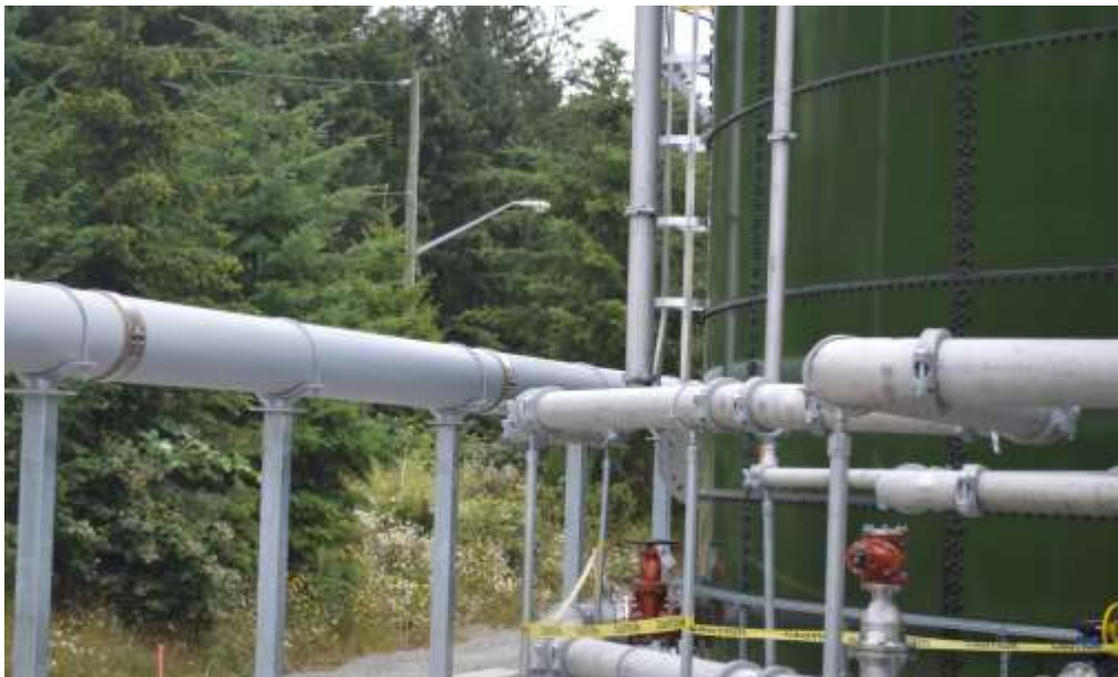
Figure 7– Residuals Treatment Facility- air ducting from Residuals Solids Tanks.
