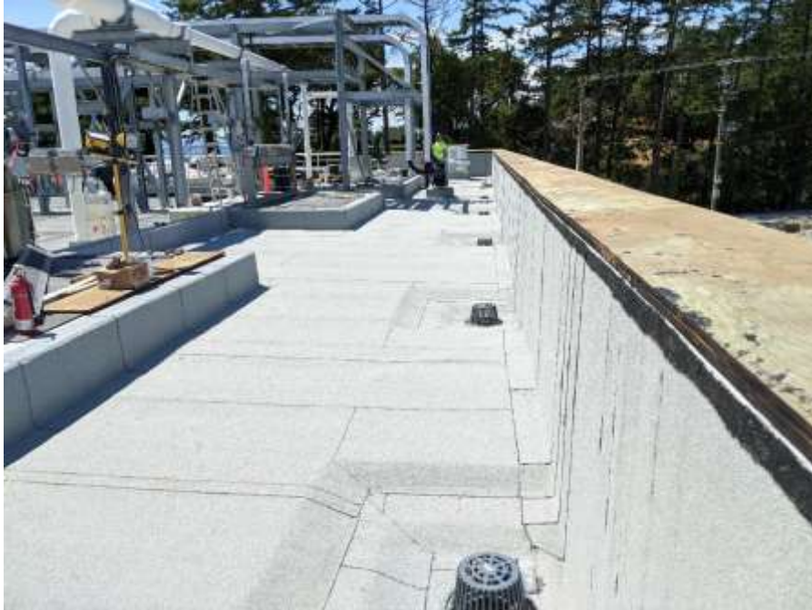
Figure 4– McLoughlin Point Wastewater Treatment Plant- Roof of north pump room, parapet flashing preparation.
