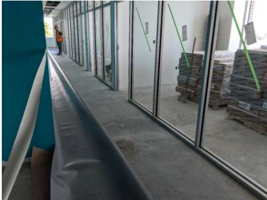
Figure 2- McLoughlin Point Wastewater Treatment Plant – Operations and Maintenance building level 2, flooring installation and glazing installed
