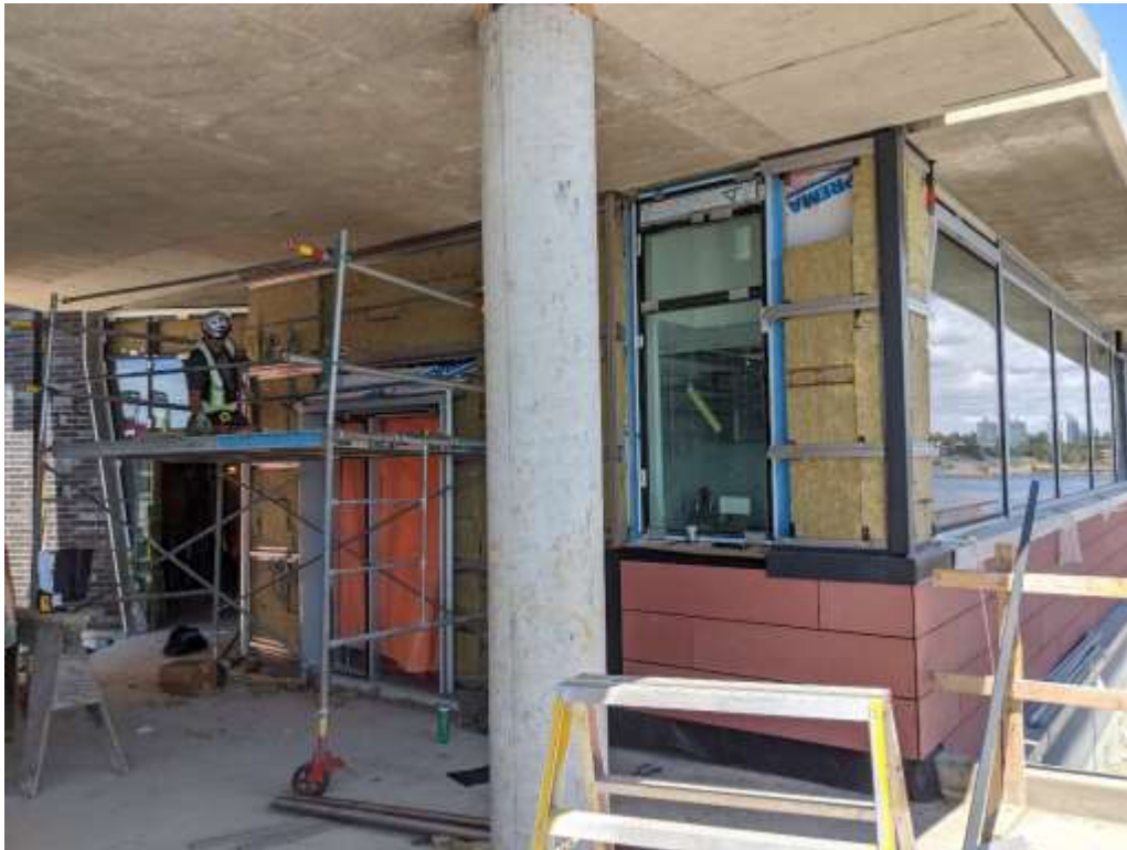
Figure 5– McLoughlin Point Wastewater Treatment Plant- Operations & Maintenance building level 1, south entrance façade insulation.
