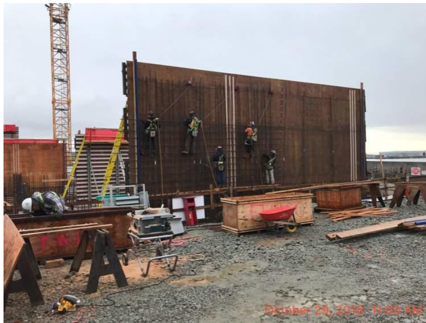
Figure 6 – McLoughlin Point Wastewater Treatment Plant: Installing rebar in biological aerated filter (BAF) wall forms.
