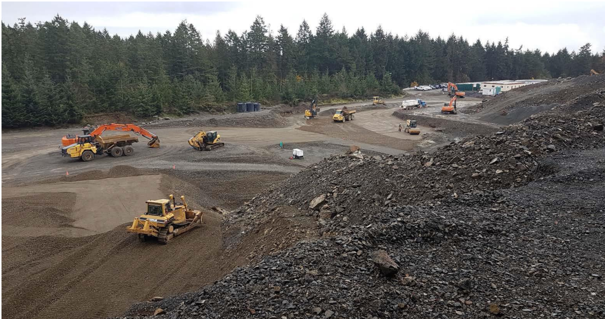
Figure 10 – Residuals Treatment Facility: Site progress looking northeast from the Hartland Landfill upper access road.
