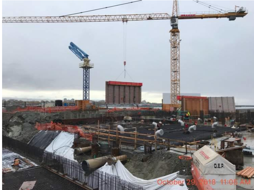
Figure 7 – McLoughlin Point Wastewater Treatment Plant: Erecting biological aerated filter (BAF) wall gang forms.
