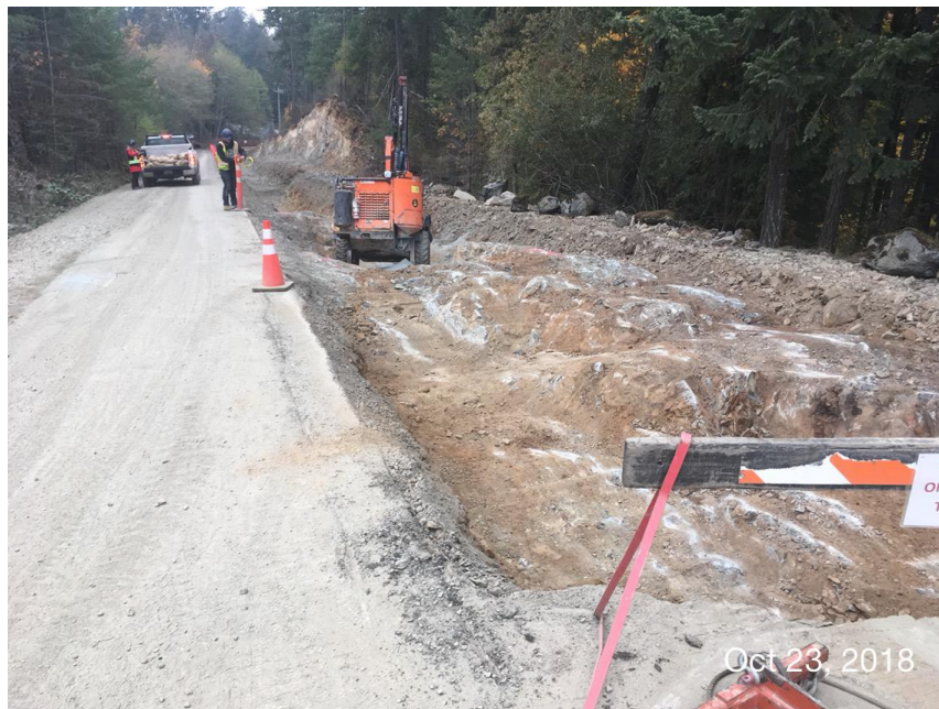
Figure 12 – Residuals Treatment Facility: Drilling rock for blasting for installation of underground utilities on main access road.
