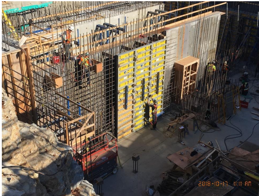
Figure 4 – McLoughlin Point Wastewater Treatment Plant: Closing tertiary wall TB-1-W11 and box out for wall TB-1-W12.
