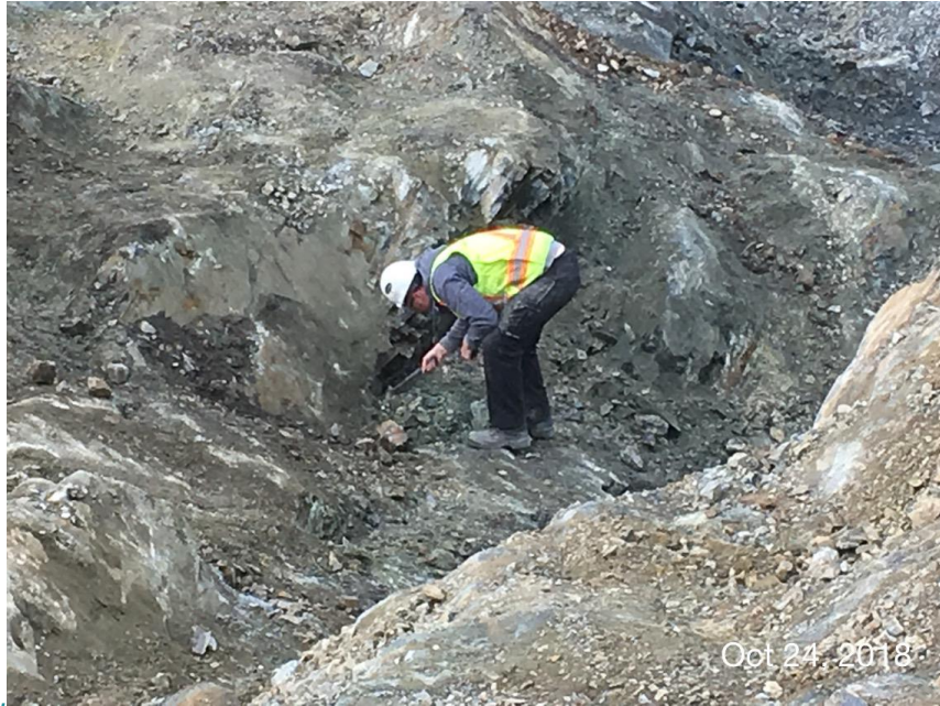
Figure 11 – Residuals Treatment Facility: Geotechnical engineer examining suitability of bedrock prior to placement of fill.
