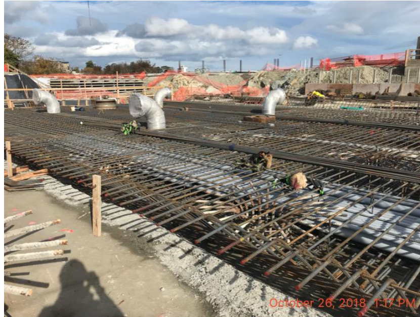
Figure 5 – McLoughlin Point Wastewater Treatment Plant: Duct bank and rebar installation in biological aerated filter (BAF) slab S5.
