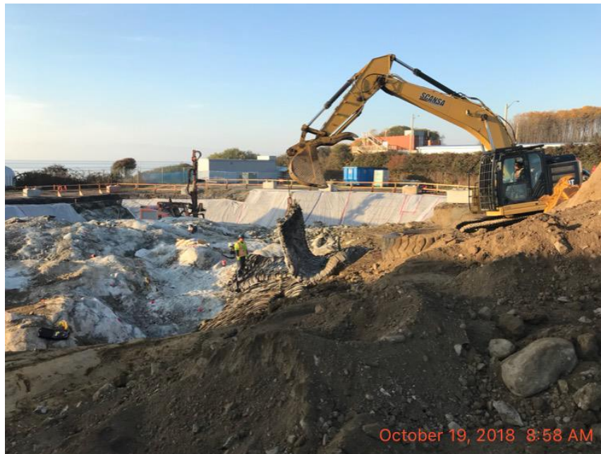
Figure 20 – Macaulay Point Pump Station: Placing of blast mat prior to blasting, excavation slope protection shown in the background.
