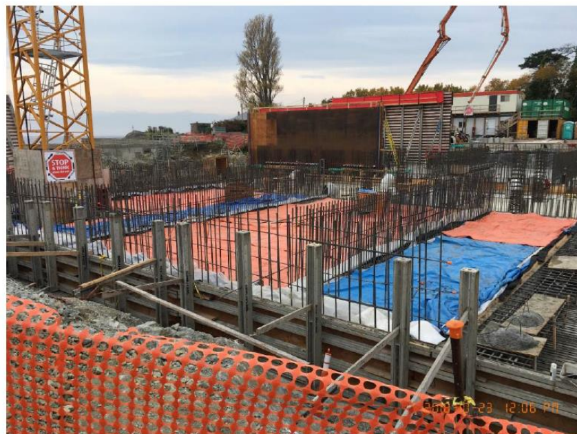
Figure 8 – McLoughlin Point Wastewater Treatment Plant: Curing of biological aerated filter (BAF) slab.
