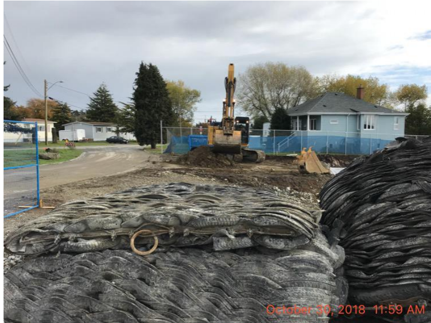
Figure 19 – Macaulay Point Pump Station: Stripping of overburden from the northeast corner of the site.
