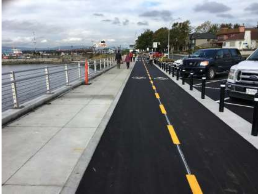
Figure 13–Clover Forcemain- Cycle track with lines painted, bollards installed and sidewalk and fence complete.
