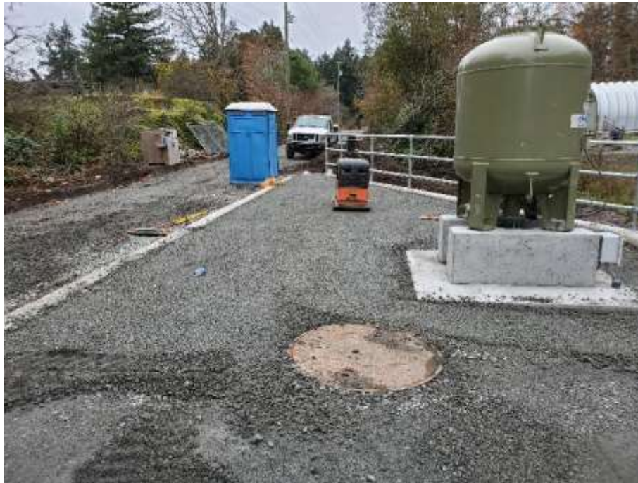
Figure 19 –Residual Solids Pump Stations – Pump Station 3- Compacted the final lift of granular material on the west end of the site
