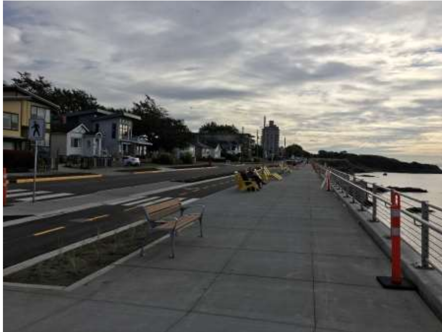
Figure 15–Clover Forcemain- Dallas road paved and benches and lounge chairs installed on sidewalk.
