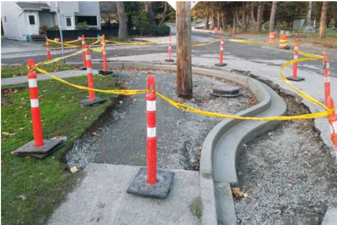
Figure 22–Trent Forcemain- Poured curbing at the intersection of Memorial Crescent and Bushby Street.
