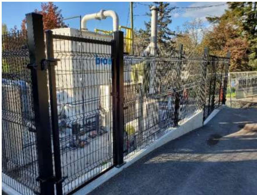
Figure 18–Residual Solids Pump Stations–Pump Station 2 – Single and double gates for the Omega fence around the odour control unit were installed
