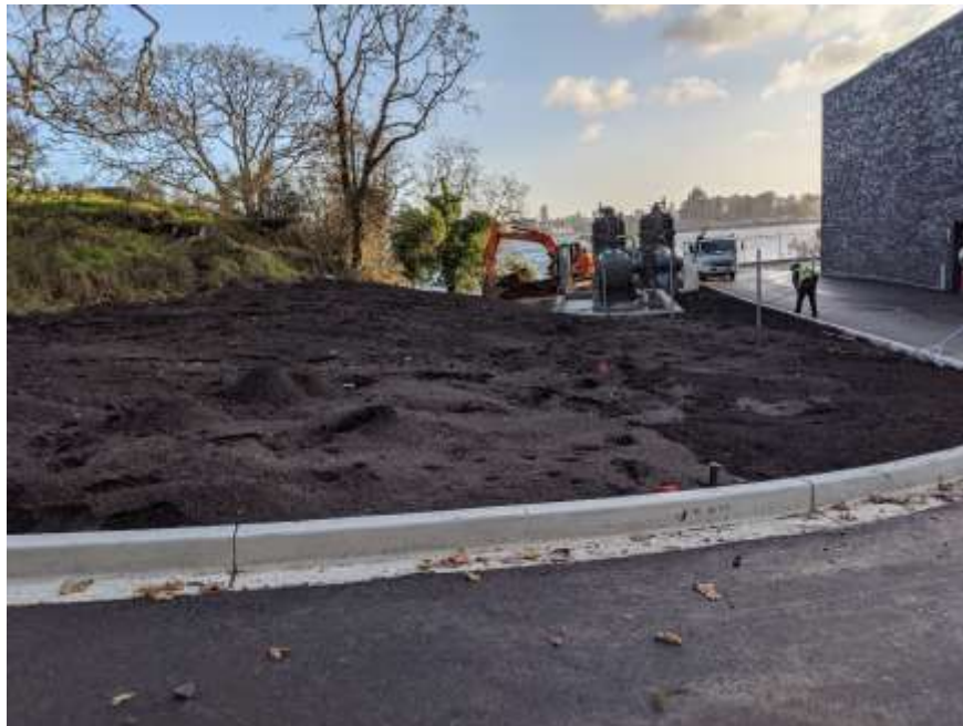
Figure 2– McLoughlin Point Wastewater Treatment Plant – Placing topsoil before planting at North Road landscape area.
