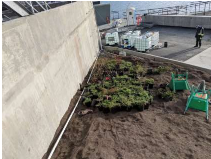
Figure 4– McLoughlin Point Wastewater Treatment Plant- Planting shrubs in planter area south of biological aerated filter cell #9.
