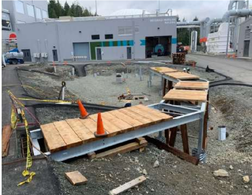
Figure 6– Residuals Treatment Facility- Construction of boardwalk in storm pond north of operations building.
