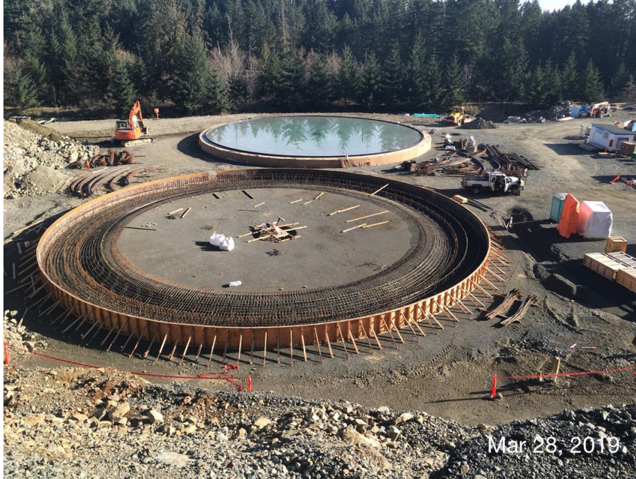
Figure 9 – Residuals Treatment Facility: digester #1 flooded for curing, and installation of reinforcing steel for first pour on digester #2
