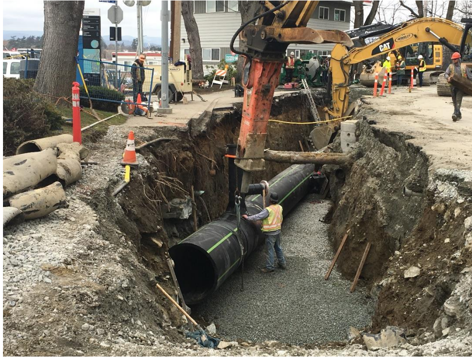
Figure 17 – Clover Forcemain: Dallas Road – Installing forcemain at Dallas Rd. and Montreal St.
