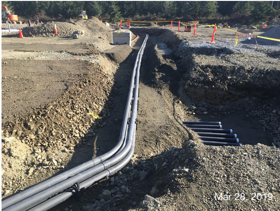
Figure 10 – Residuals Treatment Facility: installation of hydro and communications conduits east side of future centrifuge building.
