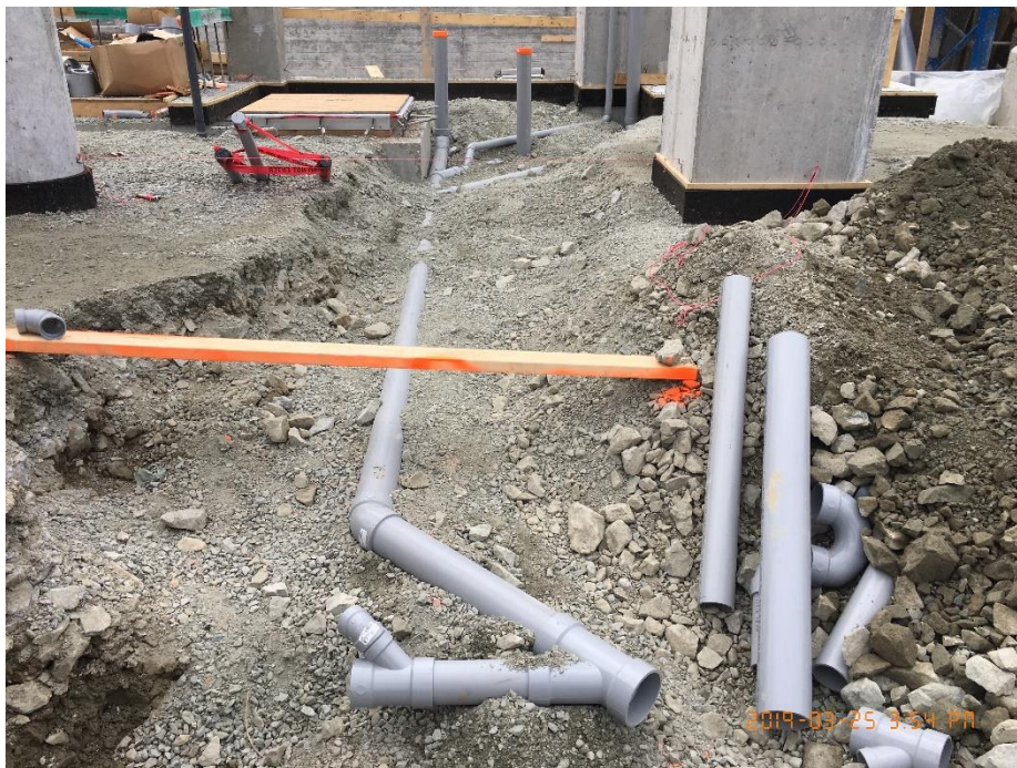
Figure 8 - McLoughlin Point Wastewater Treatment Plant: installing drain lines in operations and maintenance building slab.
