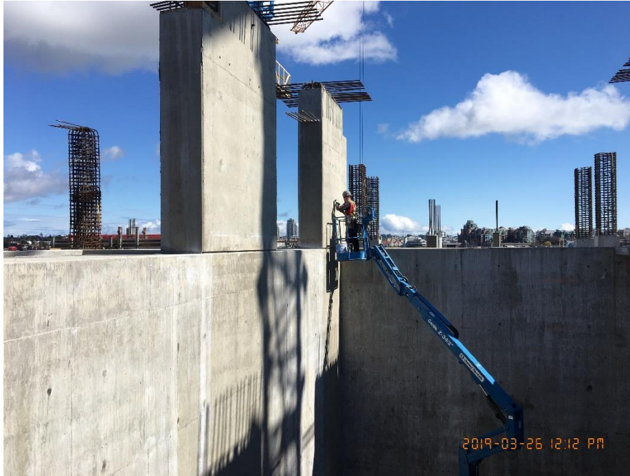
Figure 5 - McLoughlin Point Wastewater Treatment Plant: Rub and patch concrete biological aerated filter shear wall.
