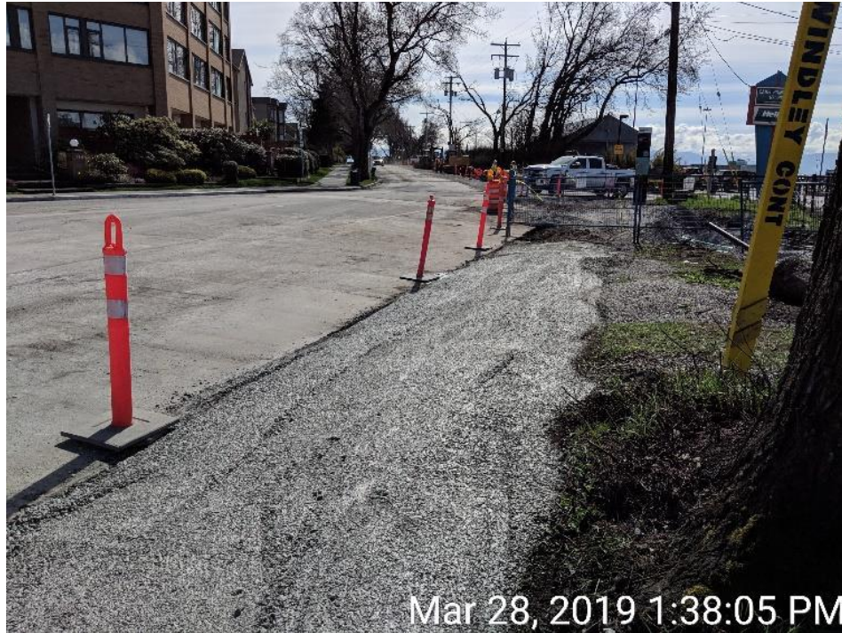
Figure 19 – Clover Forcemain: Dallas Road – Road restoration at St Lawrence and Dallas Rd..
