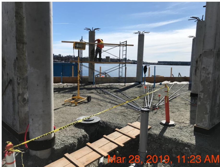
Figure 4 - McLoughlin Point Wastewater Treatment Plant: installation of electrical conduit in Lab area.
