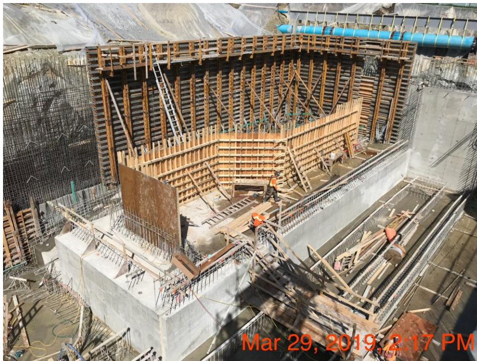
Figure 14 – Macaulay Point Pump Station: Installing rebar for the exterior wall pour and installing interior and exterior formwork.
