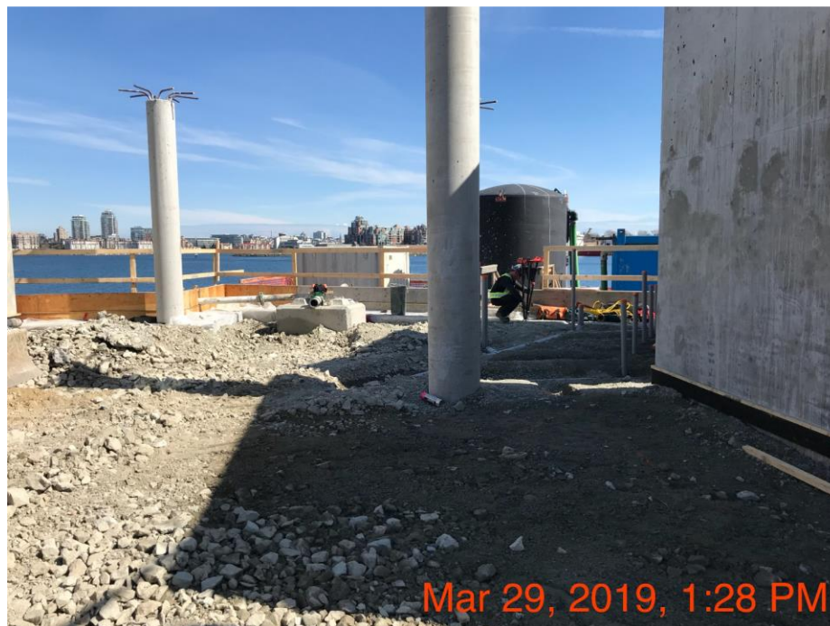
Figure 2 – McLoughlin Point Wastewater Treatment Plant: Installation of utilities in lab area changing rooms.
