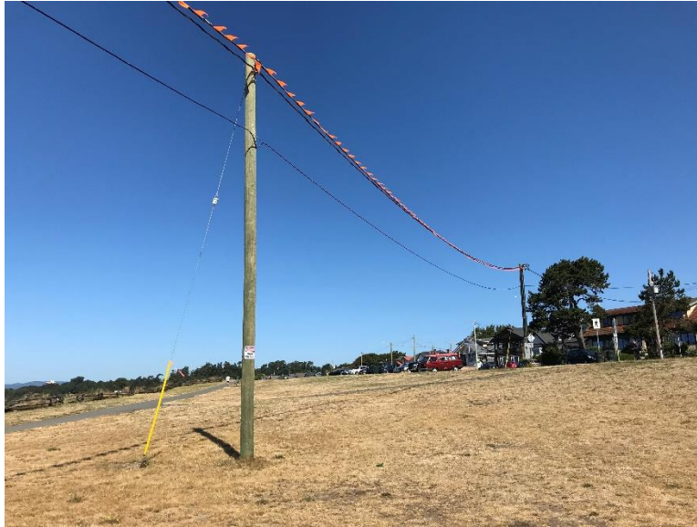
Figure 14 – Flagging and signage place on overhead power lines.
