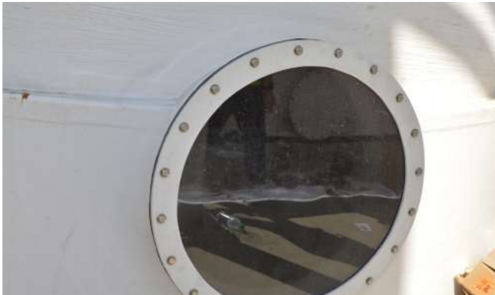
Figure 8- Residuals Treatment Facility – Wet testing and commissioning of Bio trickling Filter at Odour Control Facility.
