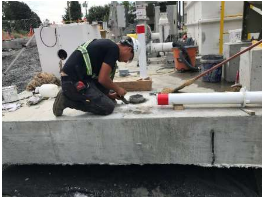
Figure 17–Residual Solids Pump Stations– Pump Station 1 –Installing bollard sleeves on the Odour Control pad.
