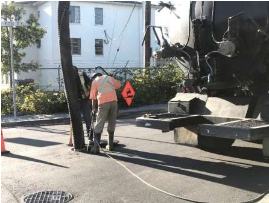
Figure 15– Residual Solids Pipes- Pressure washing manhole at Lyall Street and Peters Street.
