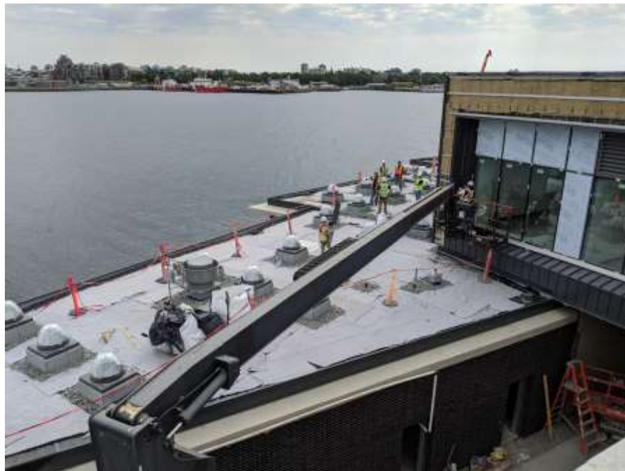
Figure 3– McLoughlin Point Wastewater Treatment Plant- operations and maintenance building north façade cladding and observation deck green roof membrane inspection.
