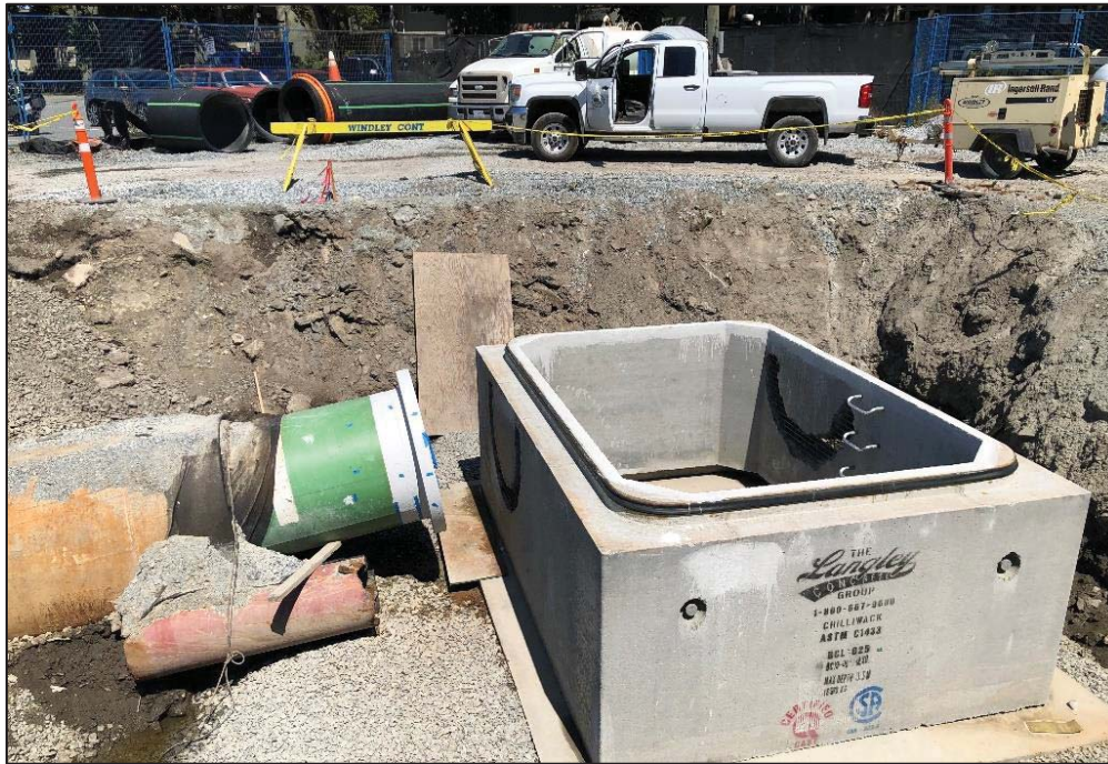
Figure 18–Clover Forcemain- Weld-Neck Flange welded and foundation and lower section of transition chamber installed.
