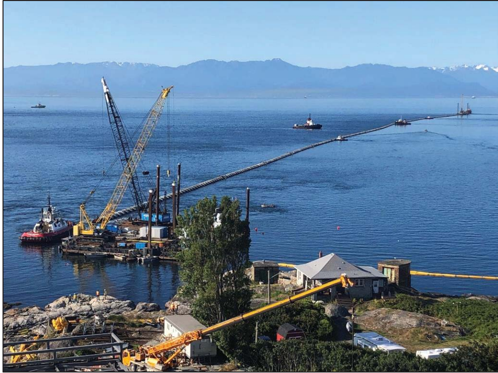
Figure 2– McLoughlin Point Wastewater Treatment Plant- Floating the marine outfall into place prior to submerging.
