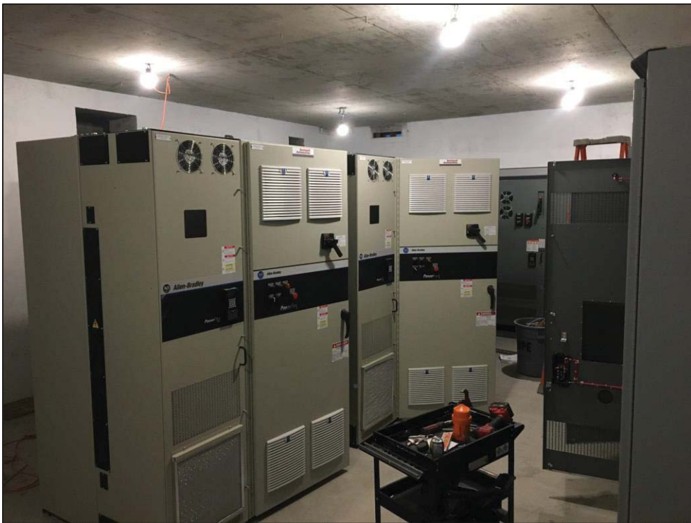
Figure 14–Clover Point Pump Station- Electrical room.
