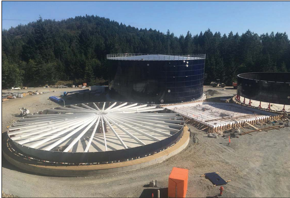
Figure 10– Residuals Treatment Facility- Site photo showing progress of Digester #2, Digester Equipment Building and Digested Solids Storage Tank.
