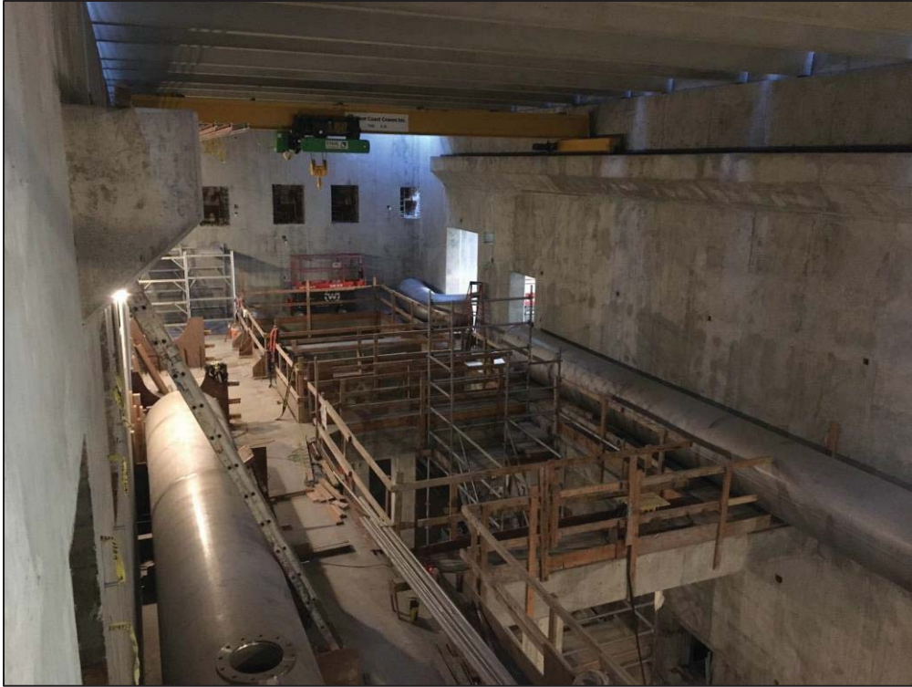
Figure 13–Clover Point Pump Station- Upper pump room.
