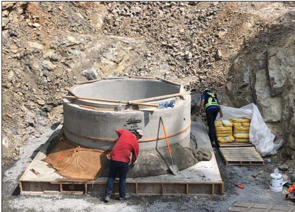
Figure 26–Residual Solids Conveyance Line- Placing and finishing non shrink grout around pump station 3 wet well.
