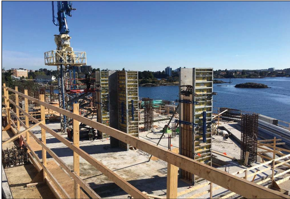
Figure 6- McLoughlin Point Wastewater Treatment Plant- Forming columns of the third level suspended slab.
