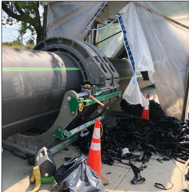
Figure 17–Macaulay Point Pump Station- Fusion welding sections of high density polyethylene pipe on Anson Street.
