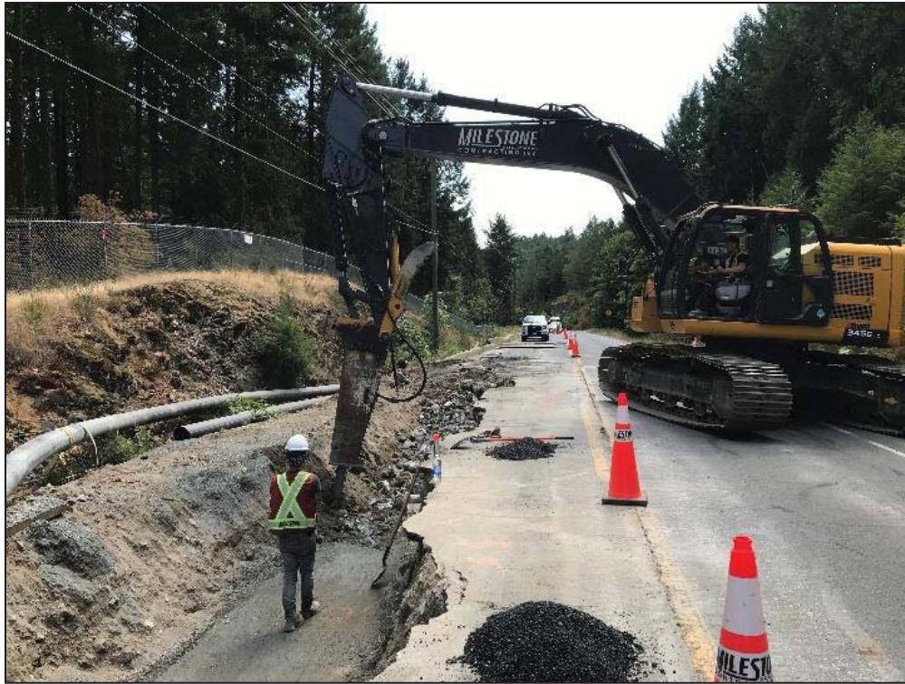
Figure 27 –Residual Solids Conveyance Line- Break rock in the trench at Willis Point Road
