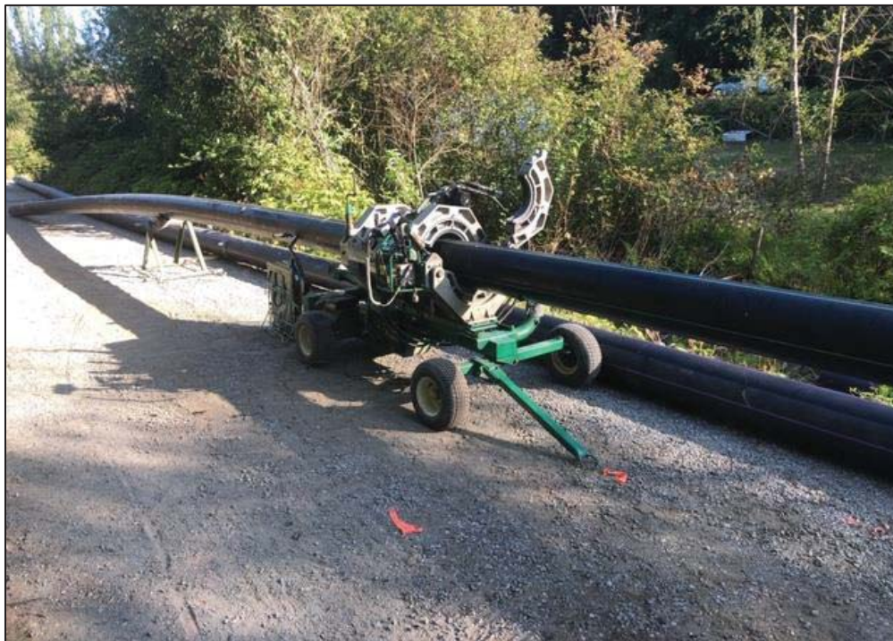
Figure 28–Residual Solids Conveyance Line- Setting up to fuse high density polyethylene pipe at pump station 2, Interurban Trail.
