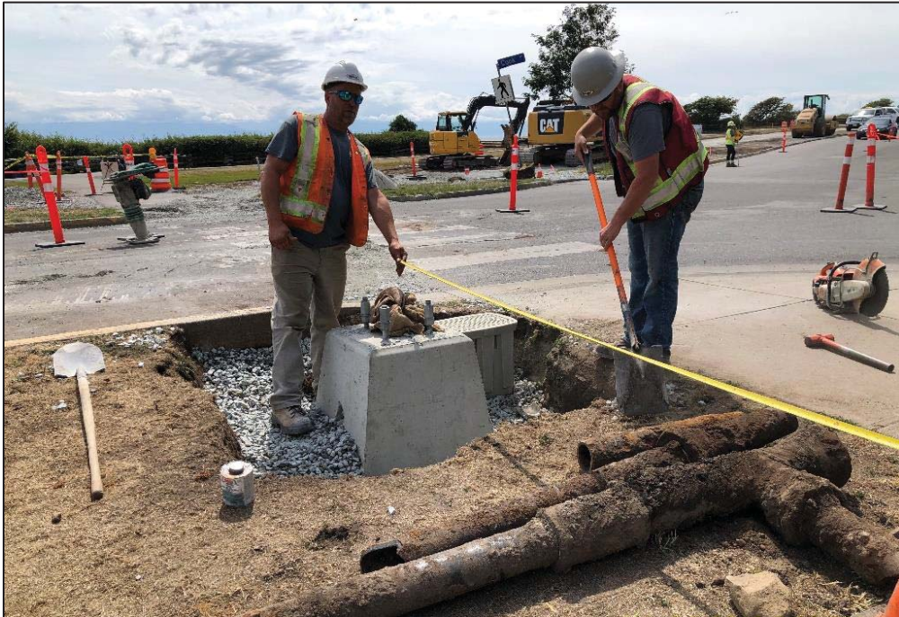
Figure 20–Clover Forcemain-- Streetlight Base and underground electrical ducting installed (Dallas at Cook St.).
