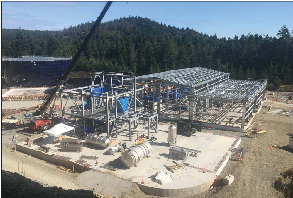
Figure 9– Residuals Treatment Facility- Site photo showing progress on Residuals Handling Building and Dryer Building.
