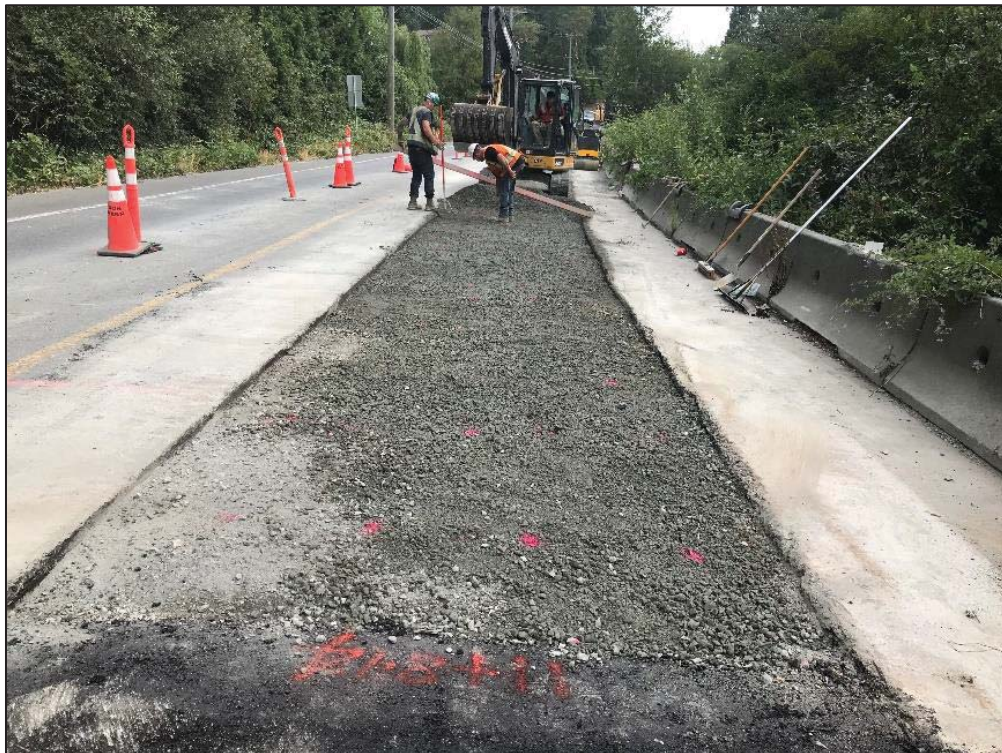
Figure 23–Residual Solids Conveyance Line- Prepping for base asphalt in segment 3 Interurban Road between Quayle Road and Goward Road.
