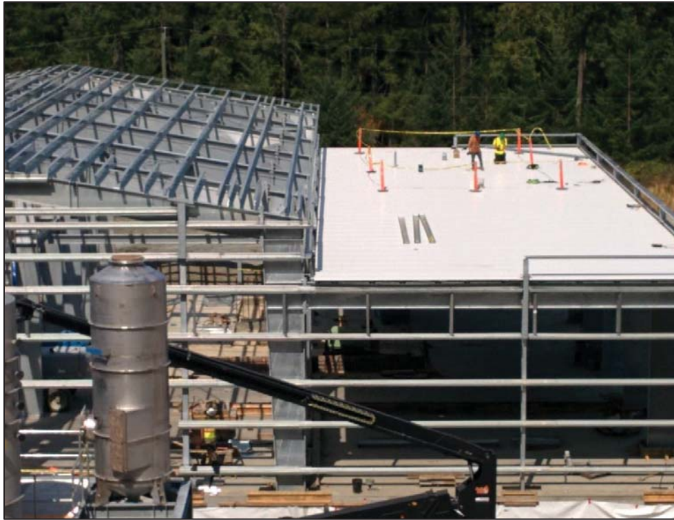
Figure 8– Residuals Treatment Facility- Residual Handling Building structural steel installation: roof bracing installation on-going.
