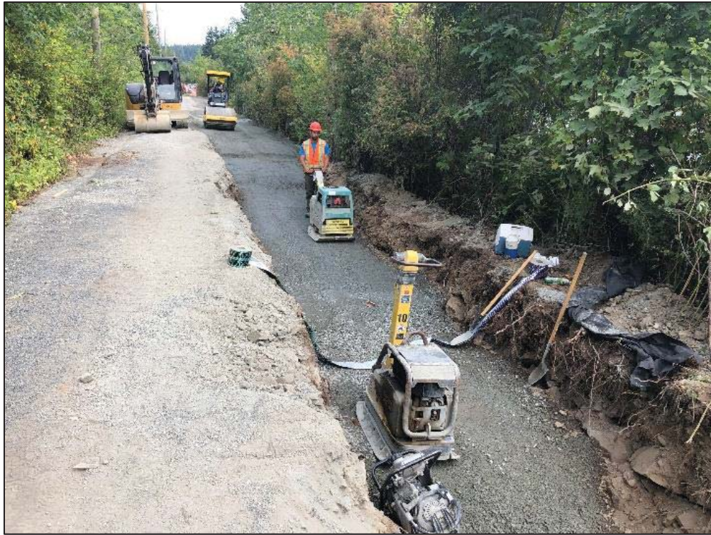
Figure 22–Residual Solids Conveyance Line- Backfilling and compaction at Interurban Trail segment 4 between Wallace Drive and Hartland Ave.
