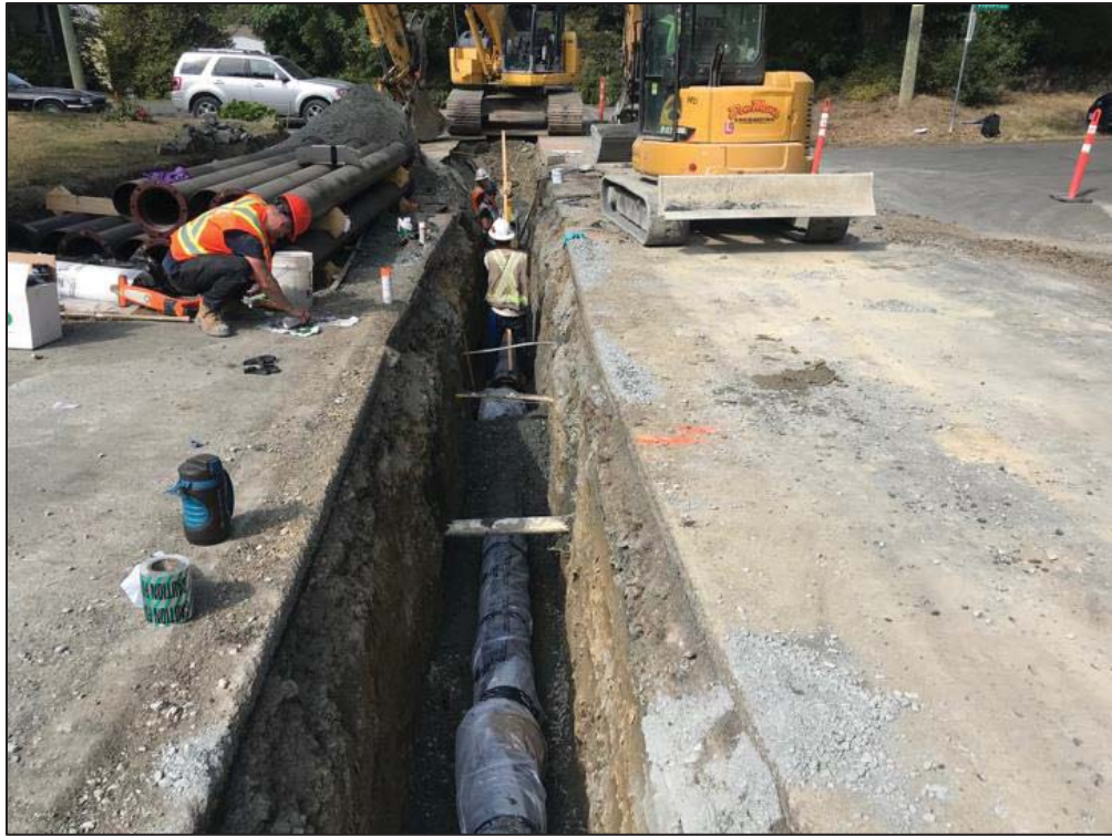
Figure 24–Residual Solids Conveyance Line- Ductile iron residual solids forcemain being installed in Segment 2, Grange Road between Violet Ave and Gardenia Court.
