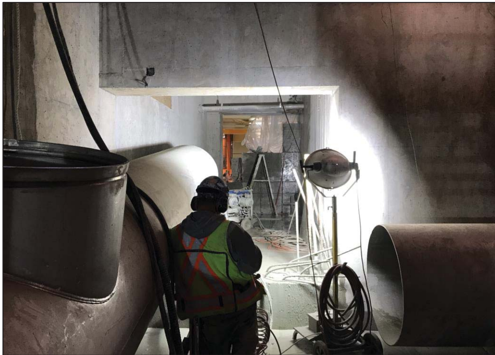
Figure 12–Clover Point Pump Station- Concrete cutting of the passageway into the existing pump station.
