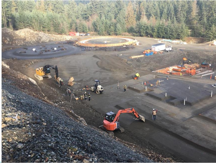
Figure 11 – Residuals Treatment Facility: overall site layout including other municipal receiving facility building slab and formwork.
