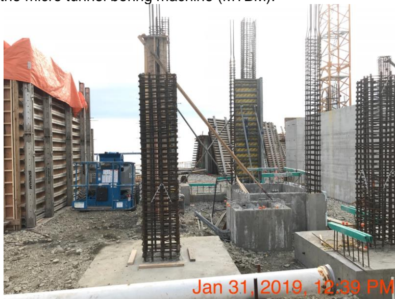
Figure 2 – McLoughlin Point Wastewater Treatment Plant: columns in operations and maintenance (O&M) building area in various stages of progress.
