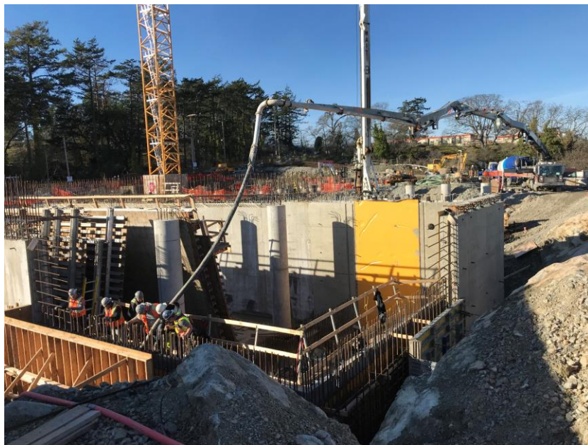
Figure 4 – McLoughlin Point Wastewater Treatment Plant: placing concrete in sludge storage tank wall.
