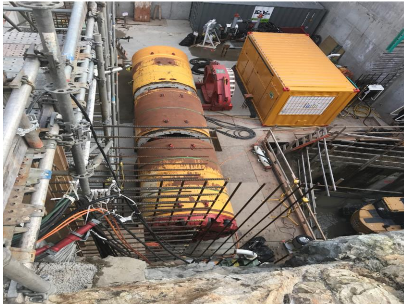
Figure 3 - McLoughlin Point Wastewater Treatment Plant: components of the micro tunnel boring machine being assembled.
