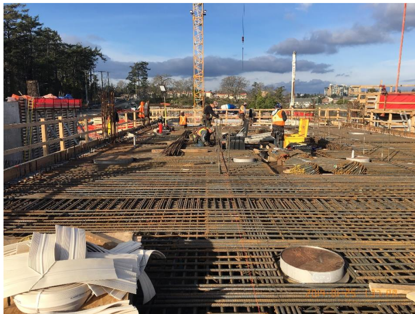
Figure 6 – McLoughlin Point Wastewater Treatment Plant: installing reinforcing steel for biological aerated filter (BAF) suspended slab.
