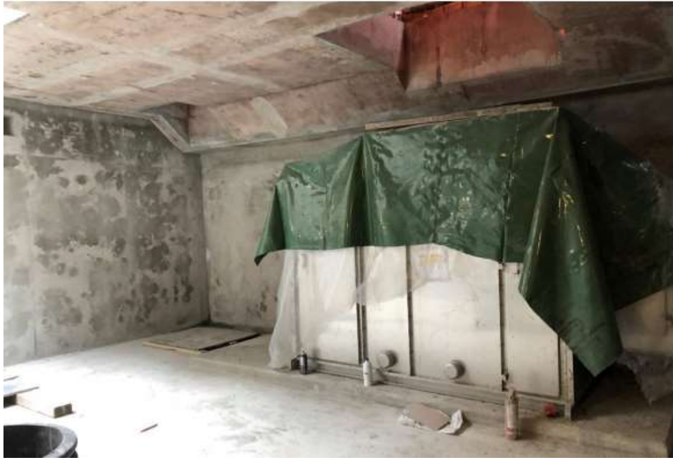
Figure 11–Arbutus Attenuation Tank- Odour Control Unit placed in Odour Control room.
