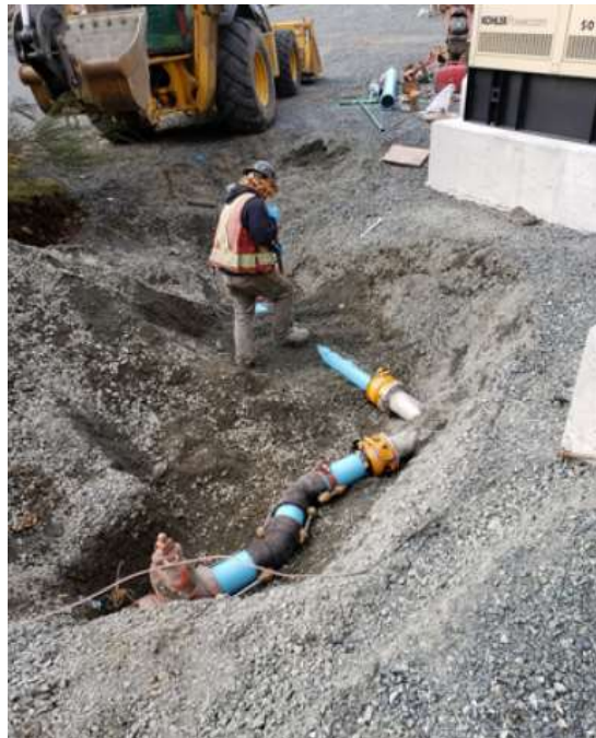
Figure 7 –Residual Solids Pump Stations – Working on watermain tie in at the Hartland Reservoir
