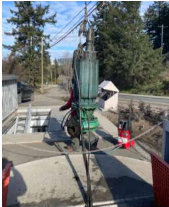
Figure 6–Residual Solids Pump Stations– Pump removed from the wet well at Pump Station 1 for inspection
