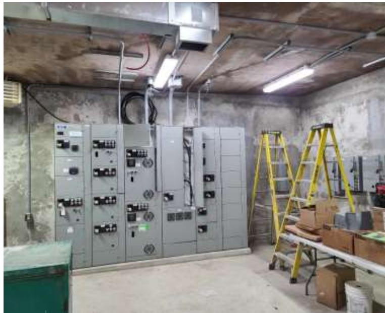
Figure 9–Arbutus Attenuation Tank- Electrical Room heating ventilation and air conditioning; and electrical installation
