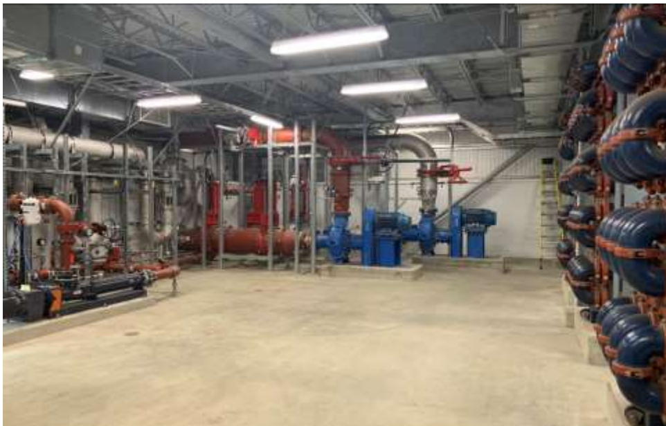
Figure 2– Residuals Treatment Facility- Digester building equipment.
