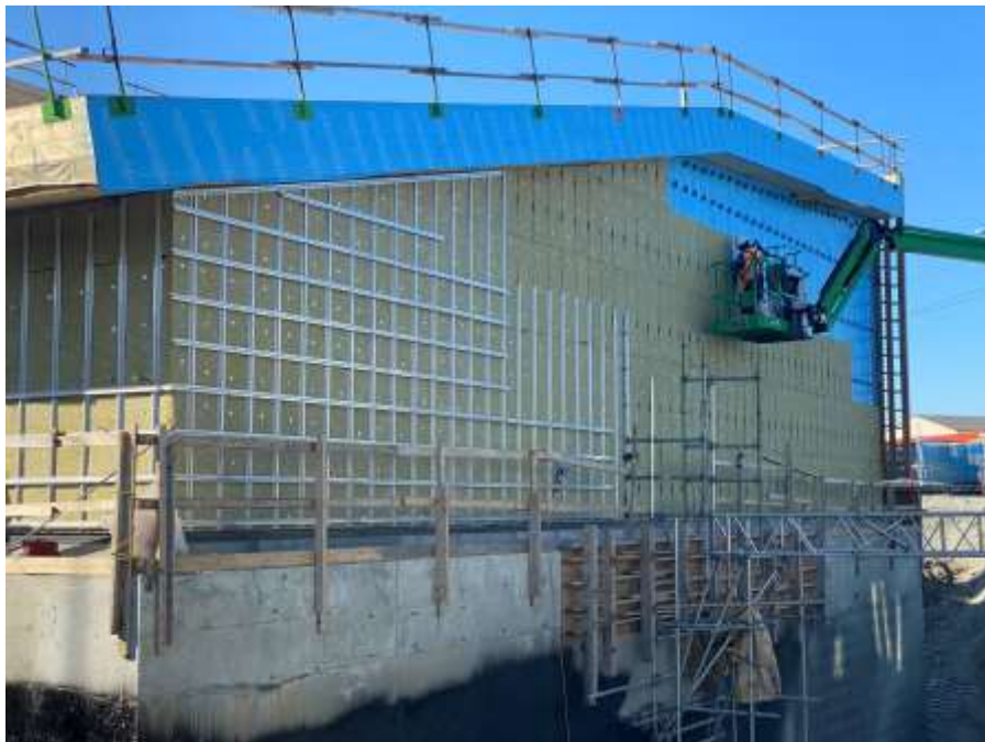
Figure 14–Macaulay Point Pump Station- Installing insulation on exterior of Cross Laminated Timber structure.
