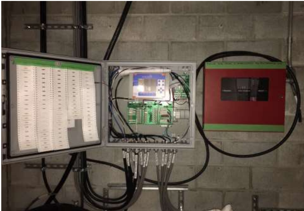
Figure 12–Clover Point Pump Station- Gas detection panel terminations
