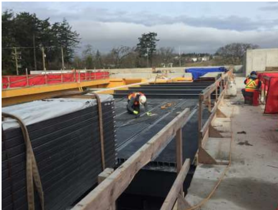
Figure 2– McLoughlin Point Wastewater Treatment Plant - installing Lamella Settler 1 roof cover and beams.
