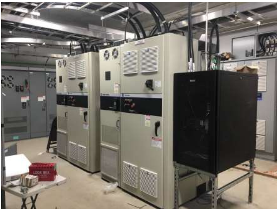
Figure 13- Clover Pump Station – Electrical room.
