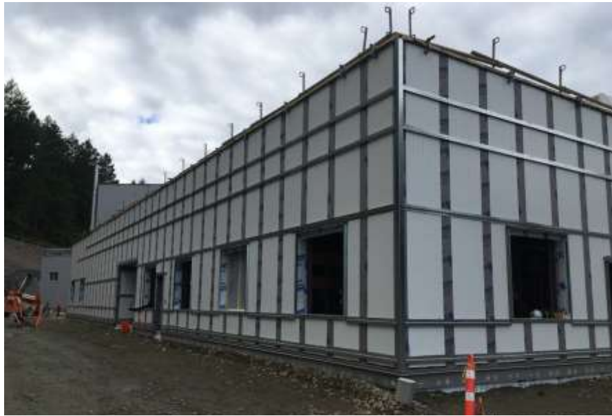
Figure 7– Residuals Treatment Facility- Operations Building installation of stand offs for exterior cladding.
