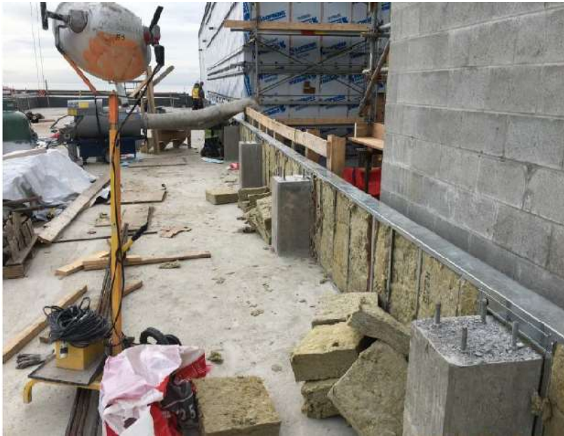
Figure 3- McLoughlin Point Wastewater Treatment Plant- Insulating parapet on Operations and Maintenance roof.
