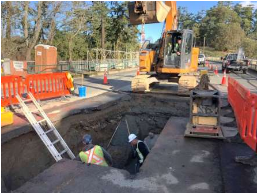
Figure 20– Residual Solids Pipes-Installation of line and drain valves on Tillicum Road north of the Tillicum Bridge.
