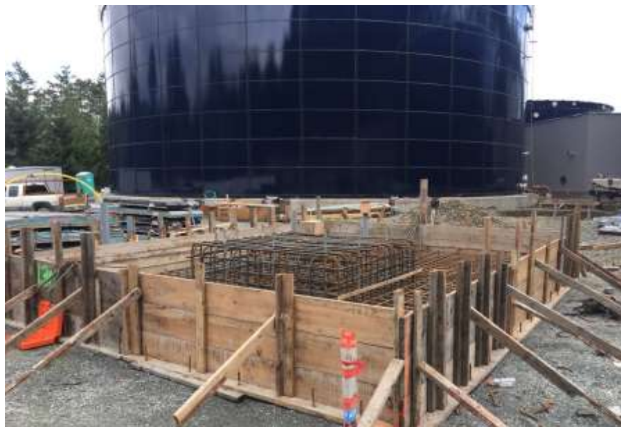
Figure 10– Residuals Treatment Facility – Form work and rebar installed for waste gas burner slab.
