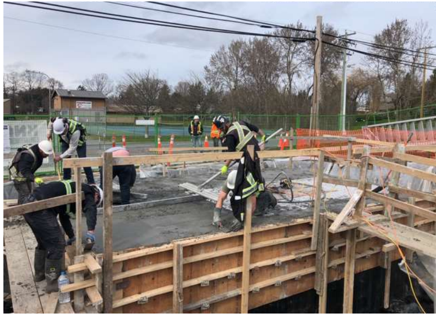
Figure 25 –Residual Solids Pump Stations - Marigold valve chamber finishing concrete of suspended slab pour.
