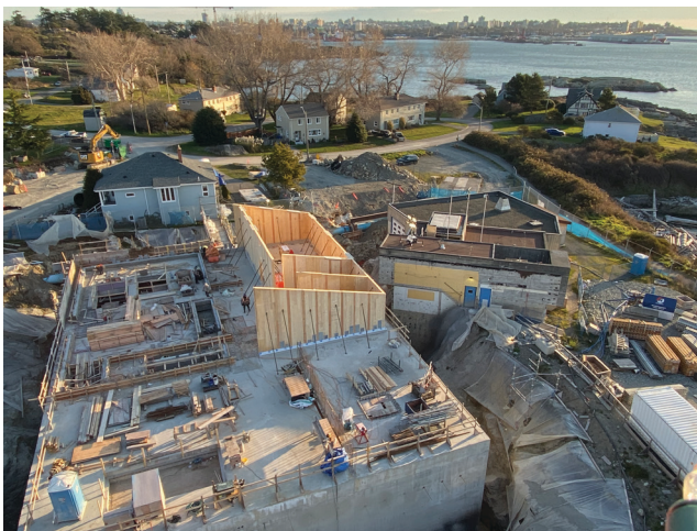
The above-ground timber structure is being constructed at Macaulay Point Pump Station.
