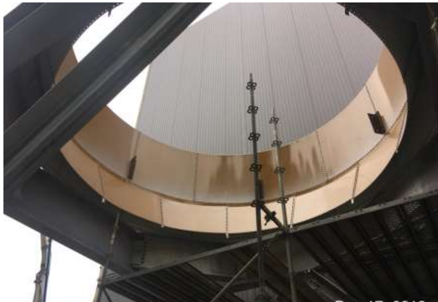
Figure 8– Residuals Treatment Facility- Product storage silo being constructed on south side of dryer building.
