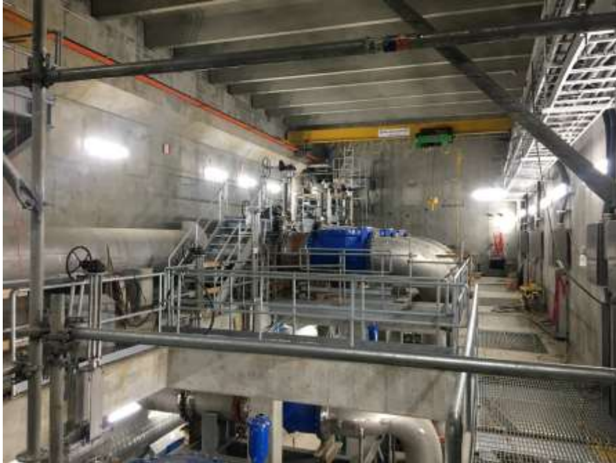
Figure 11–Clover Point Pump Station- Upper pump room looking south.
