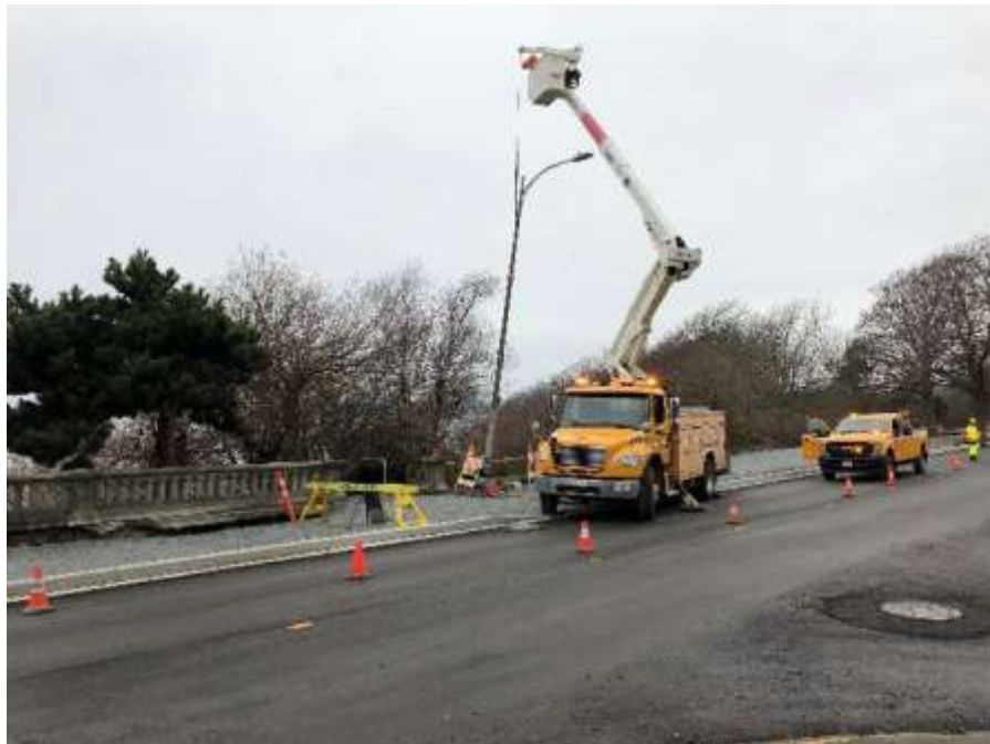
Figure 19–Clover Forcemain– Lamp standard installation near Paddon Ave.
