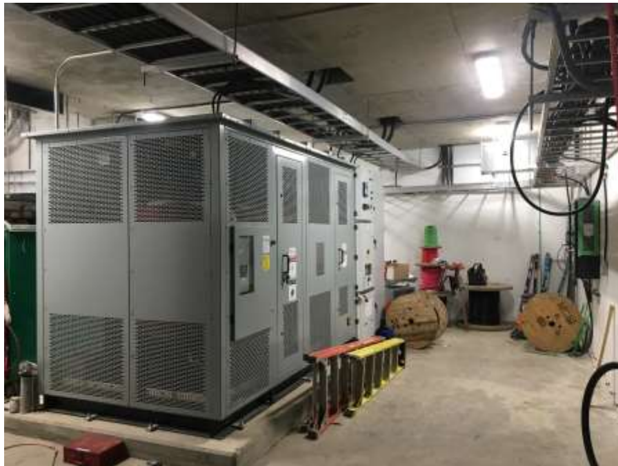
Figure 12–Clover Point Pump Station- Transformer room.
