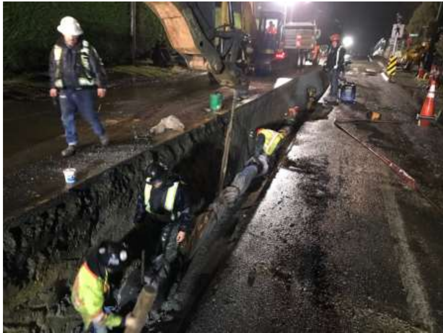
Figure 23--Residual Solids Pipes-- Ductile iron pipe installation on Interurban Rd during night work.
