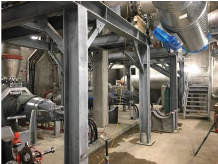
Figure 14- Clover Pump Station - Lower pump room looking north.
