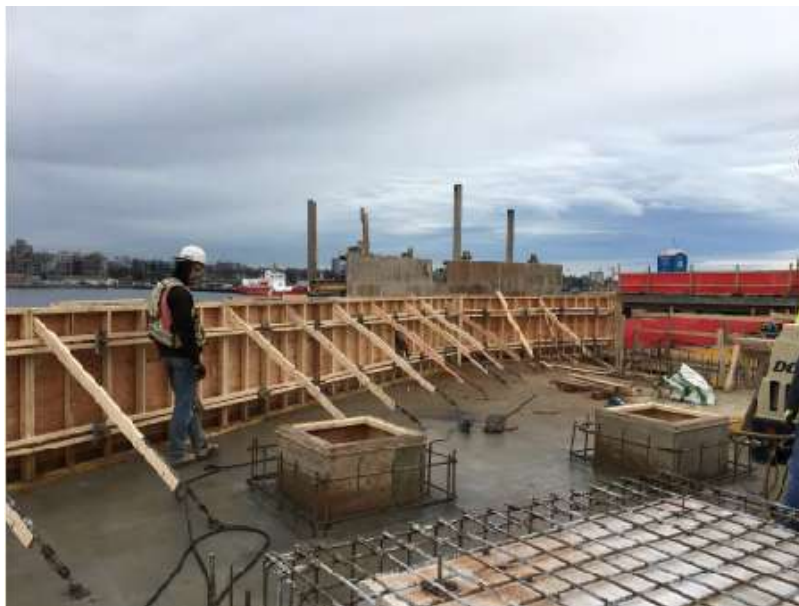
Figure 5– McLoughlin Point Wastewater Treatment Plant-Fforming odour control roof parapet and roof penetration curbs.
