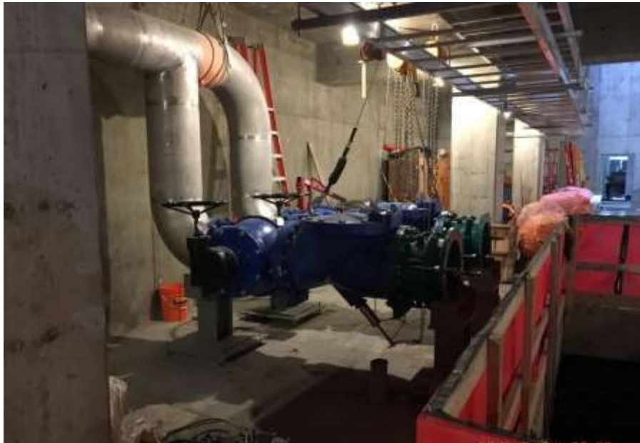
Figure 4– McLoughlin Point Wastewater Treatment Plant- Installation of control valves and check valves for backwash piping.
