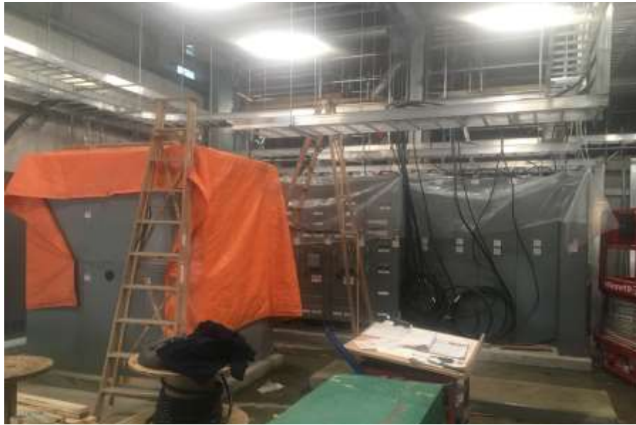
Figure 10– Residuals Treatment Facility -Installation of motor control centres and switchgear in Residuals Handling Building electrical room.
