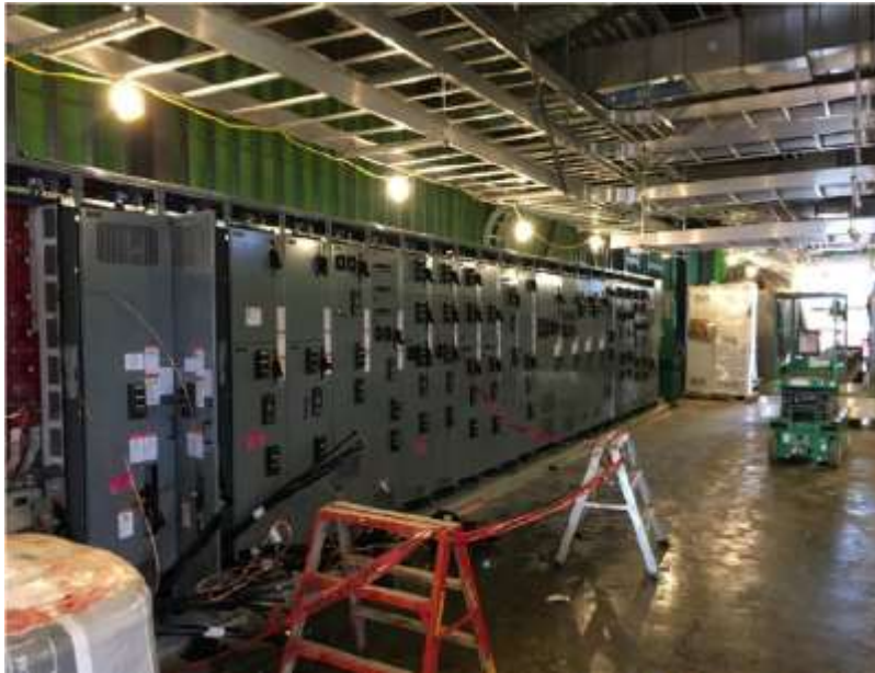
Figure 6– McLoughlin Point Wastewater Treatment Plant- Landing electrical feeds in Motor Control Centres.
