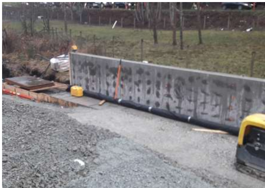
Figure 27–Residual Solids Pump Stations – Pump Station 2 – installation of drain tile at retaining wall.
