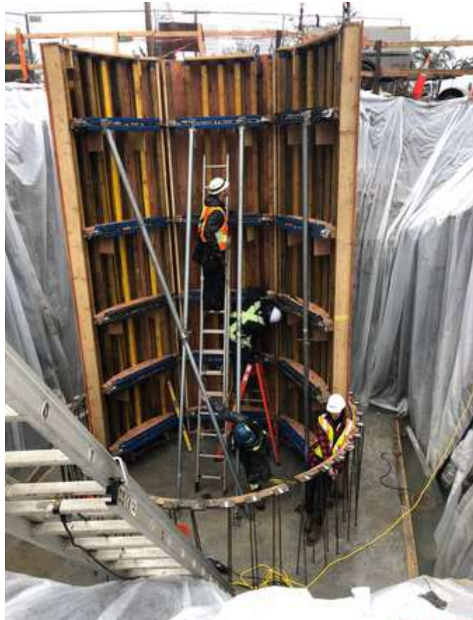
Figure 25–Residual Solids Pump Stations – Pump Station 1 – installation of formwork for the wet well.
