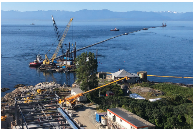
The outfall pipe being installed in July is 2.25m in diameter and 1.92km long.
