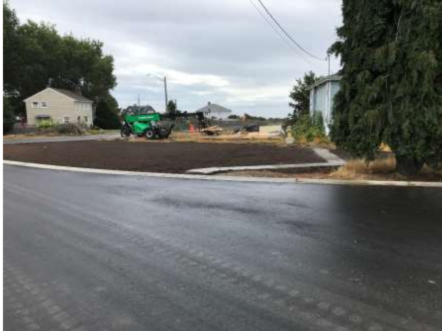
Figure 13—Macaulay Point Pump Station- Clean up and landscaping east of the blue house.
