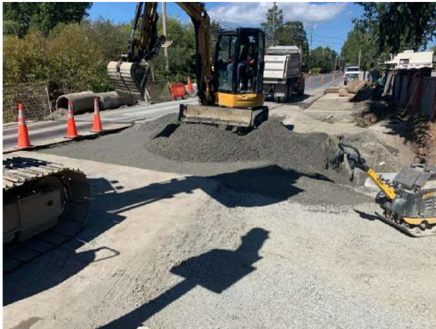
Figure 16– Residual Solids Pipes- Peers Creek – Base gravel being placed and graded over culverts.
