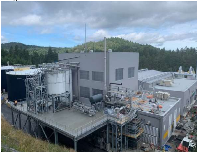
Figure 6– Residuals Treatment Facility- Dryer building and residuals handling building.
