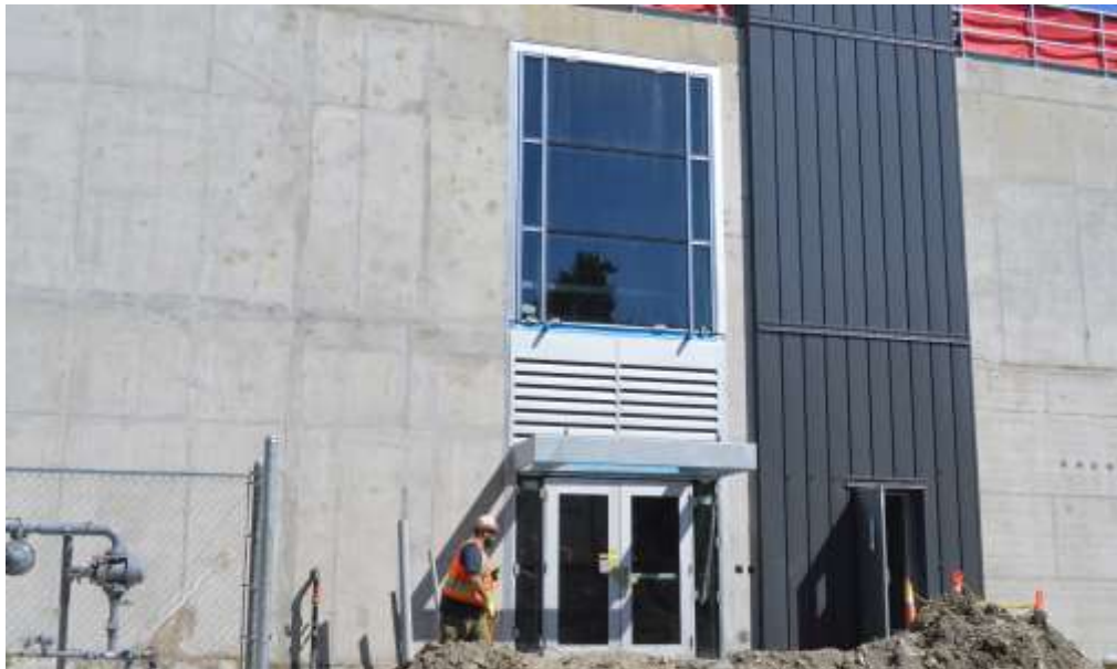
Figure 5- McLoughlin Point Wastewater Treatment Plant- Louvers installed at west entrance above doorway.
