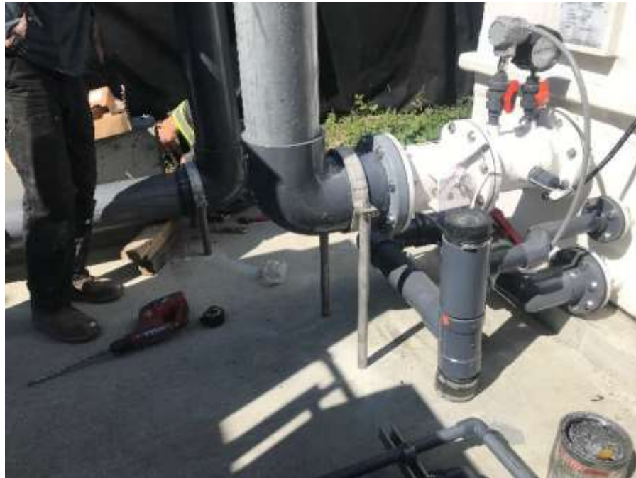
Figure 19 –Residual Solids Pump Stations – Pump Station # 1: installing pipe stands on the Odour Control Unit vent piping.
