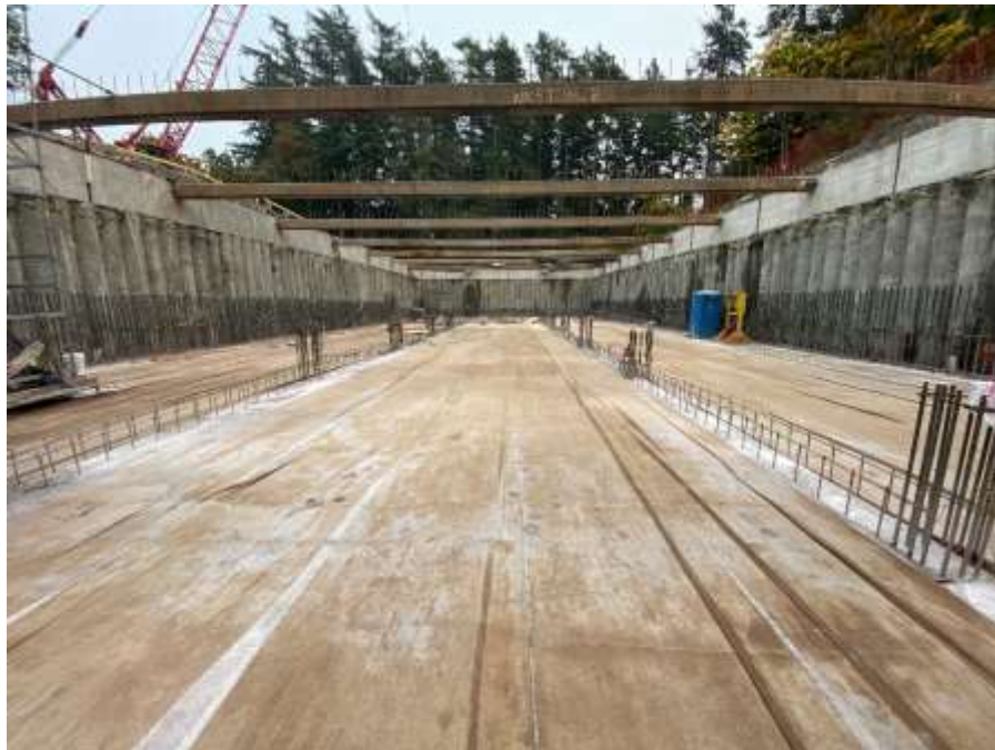
Figure 21–Arbutus Attenuation Tank- slab pour complete and covered with wet blankets for curing.
