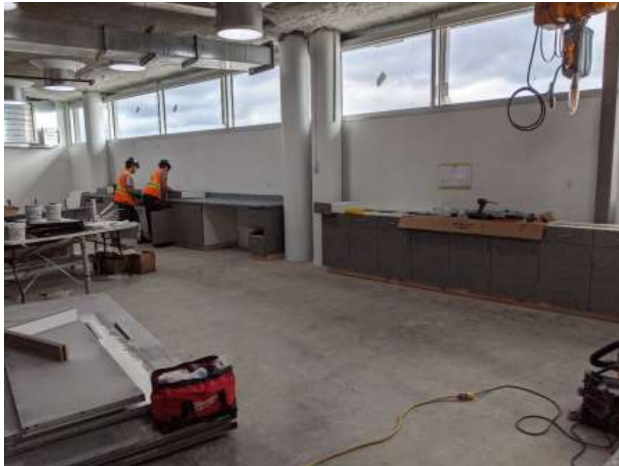
Figure 4- McLoughlin Point Wastewater Treatment Plant- Cabinet installation in workshop – Operations and Maintenance Level 1.
