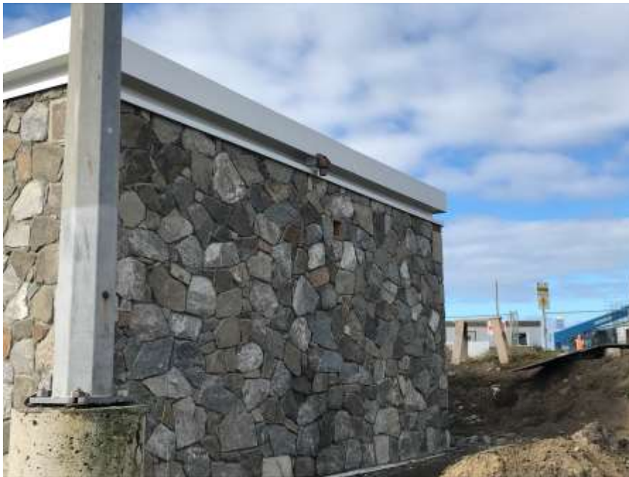
Figure 9—Clover Point Pump Station- Stonework masonry completed on exterior of public washroom.
