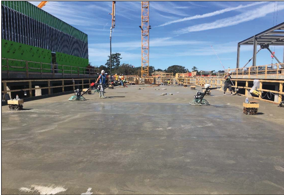
Figure 5- McLoughlin Point Wastewater Treatment Plant- Pouring and finishing BAF blower room slab.
