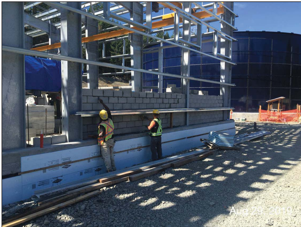
Figure 8- Residuals Treatment Facility- Masonry block wall construction ongoing in residuals handling building.
