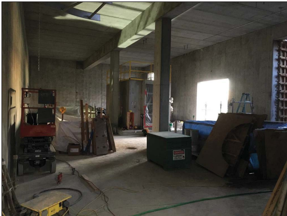
Figure 13–Clover Point Pump Station- odour control and screening room.
