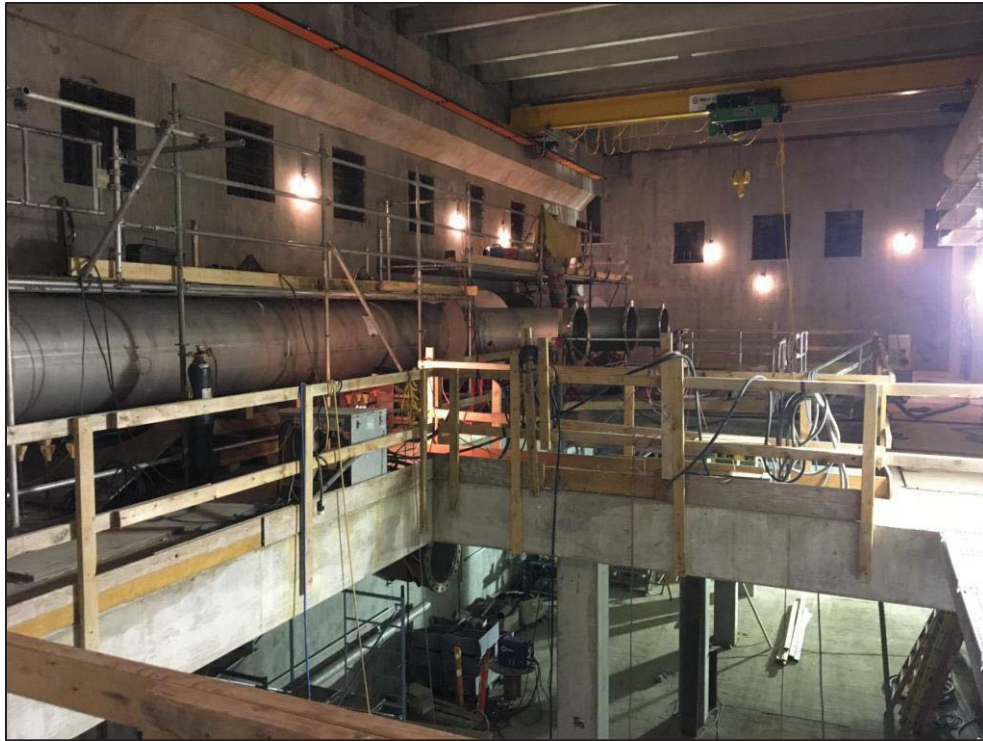
Figure 12–Clover Point Pump Station- upper pump room south view.
