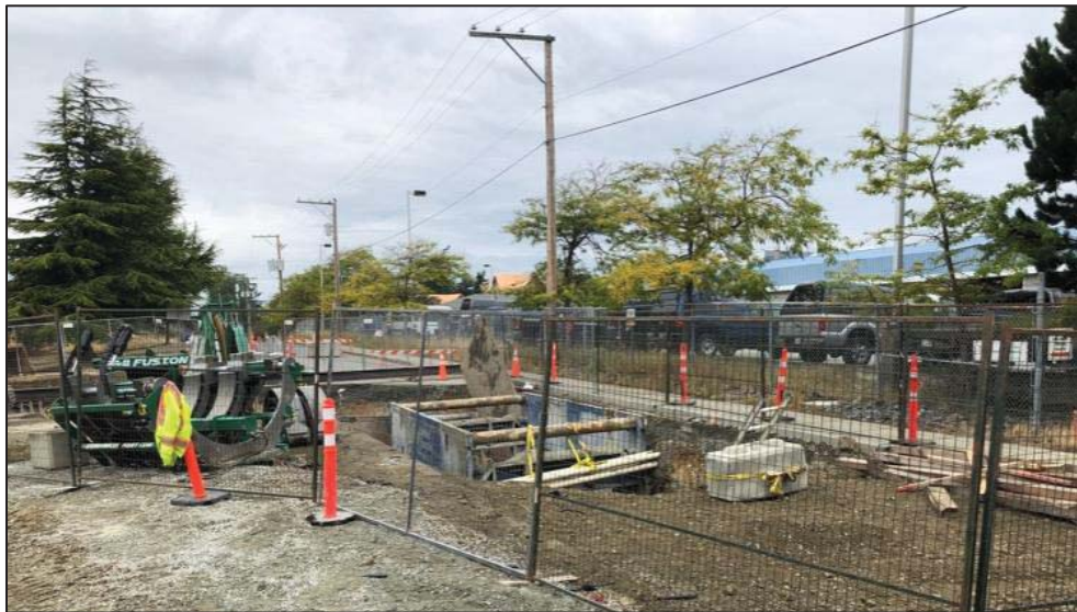
Figure 15–Macaulay Point Pump Station- Macaulay forcemain progressing east on Bewdley St to Peter St.
