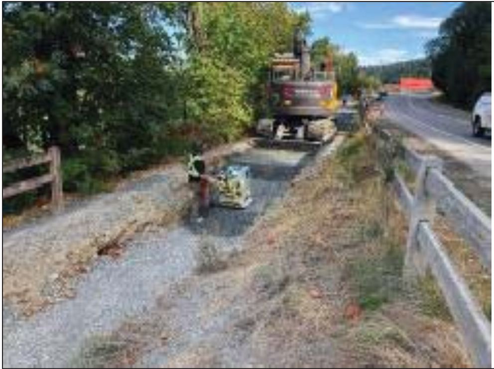
Figure 22–Residual Solids Conveyance Line- Ongoing backfill and compaction on Interurban Trail running parallel with West Saanich Road.
