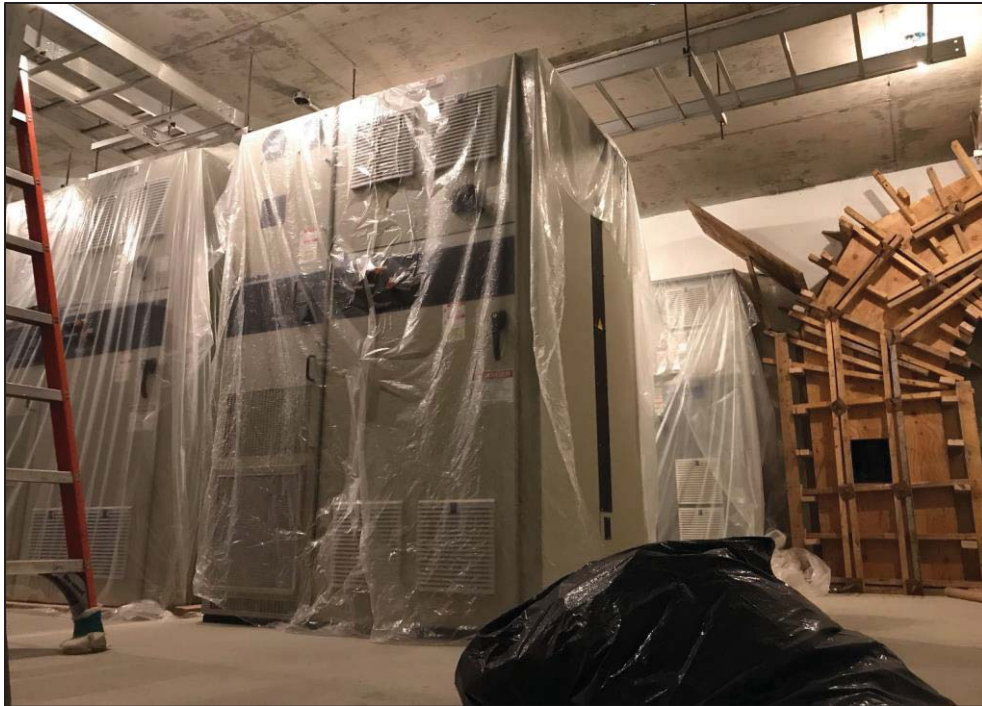
Figure 14-Clover Point Pump Station- inside the electrical room.
