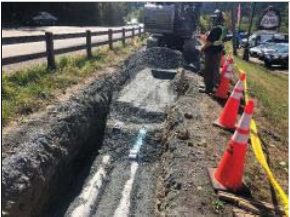
Figure 23–Residual Solids Conveyance Line- Ongoing backfill and compaction in front of Red Barn Market.
