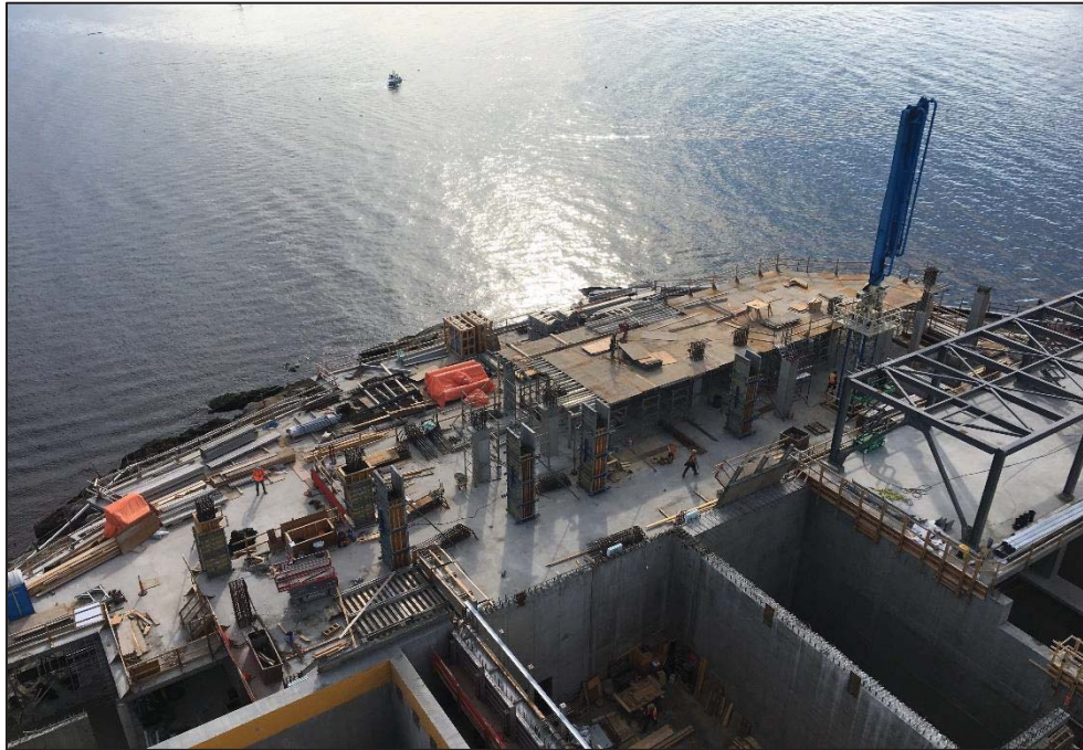
Figure 3- McLoughlin Point Wastewater Treatment Plant- View of operations and maintenance building from tower crane B.
