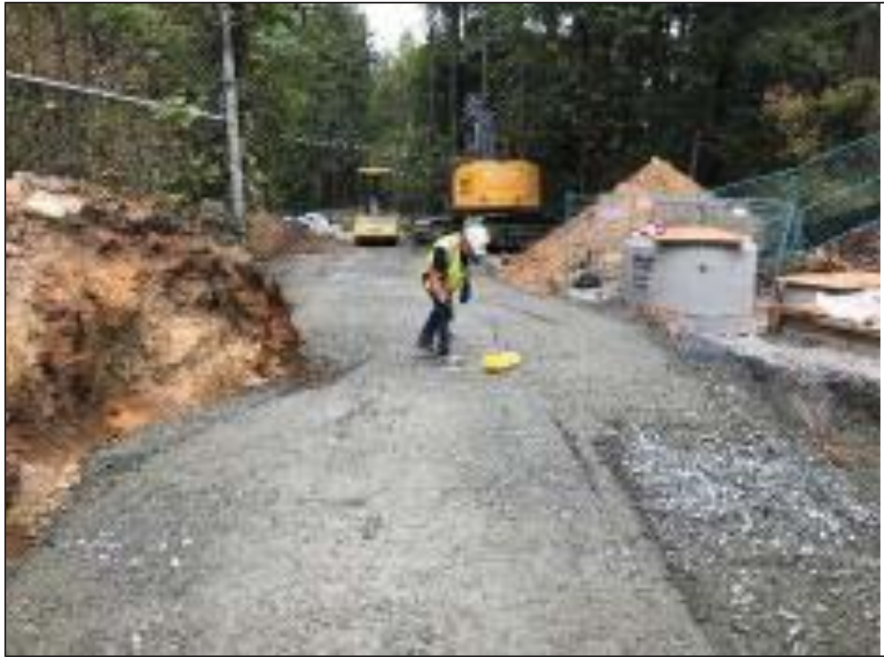
Figure 25–Residual Solids Pump Stations and Bridge Crossings –performing a compaction test on Pump Station #2 haul road.
