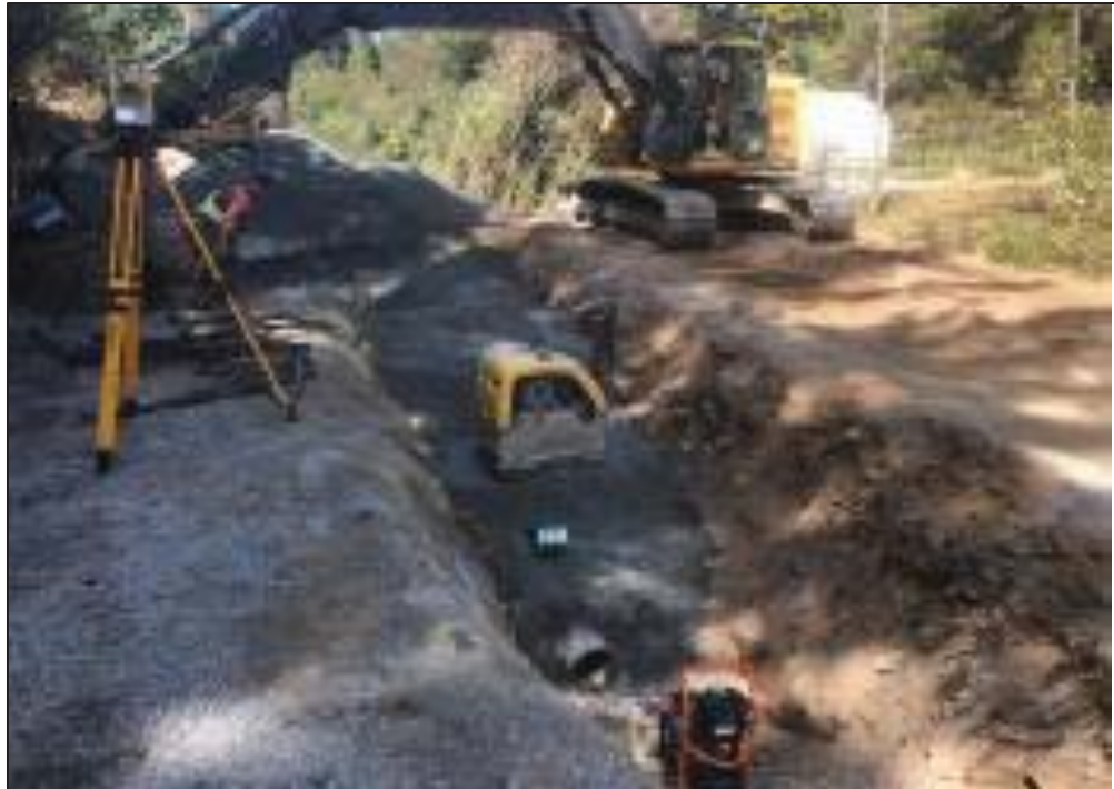
Figure 27–Residual Solids Pump Stations and Bridge Crossings – Backfilling the Residual Solids Forcemain at Pump Station 1 in lifts.
