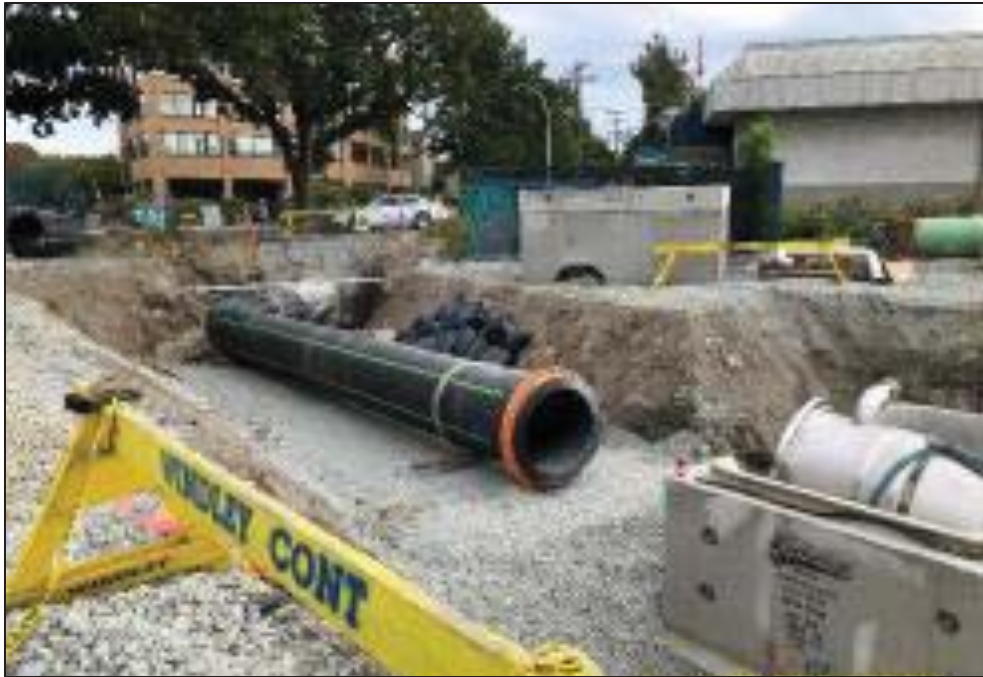
Figure 17–Clover Forcemain-Ogden Point - Weld-Neck Flange and transition chamber.
