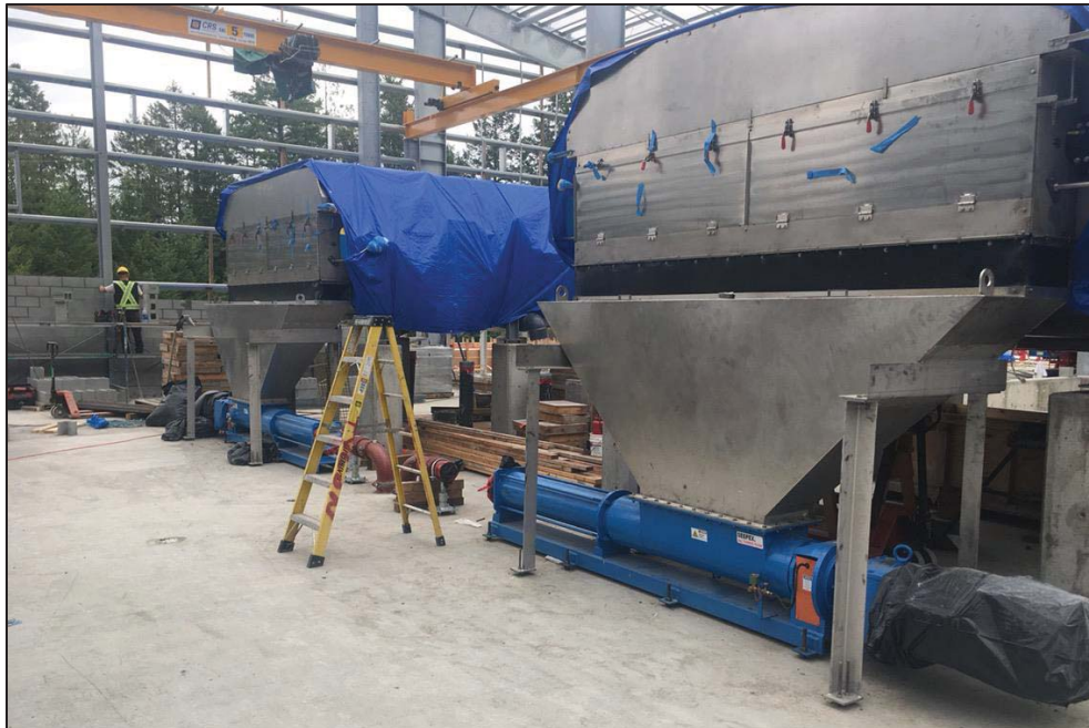
Figure 10- Residuals Treatment Facility- Installation of screw conveyors and mechanical piping for gravity belt thickeners.
