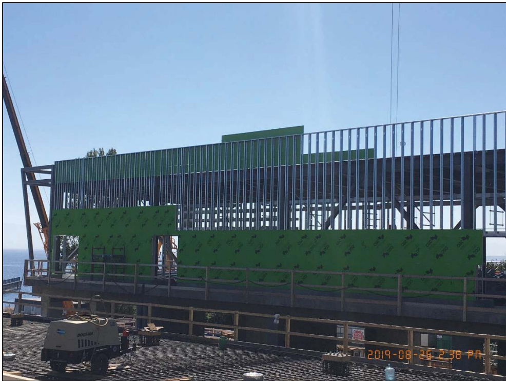
Figure 6- McLoughlin Point Wastewater Treatment Plant- Installing exterior sheathing for electrical room and room parapet.
