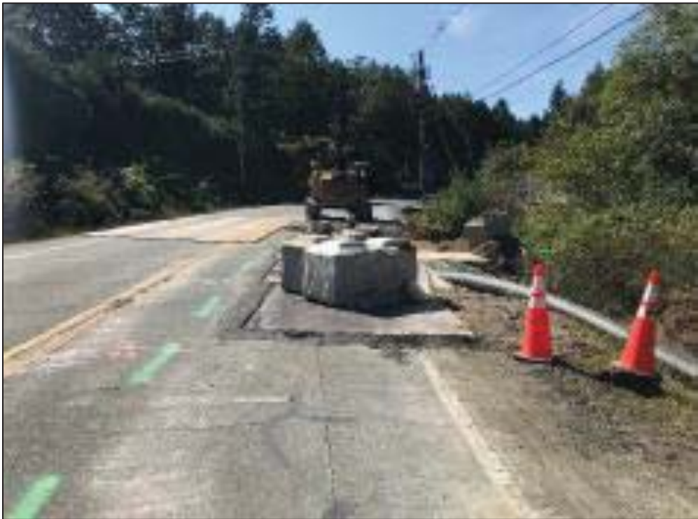
Figure 26 –Residual Solids Pump Stations and Bridge Crossings- Adjusting and stabilizing road plates on Willis Point Road
