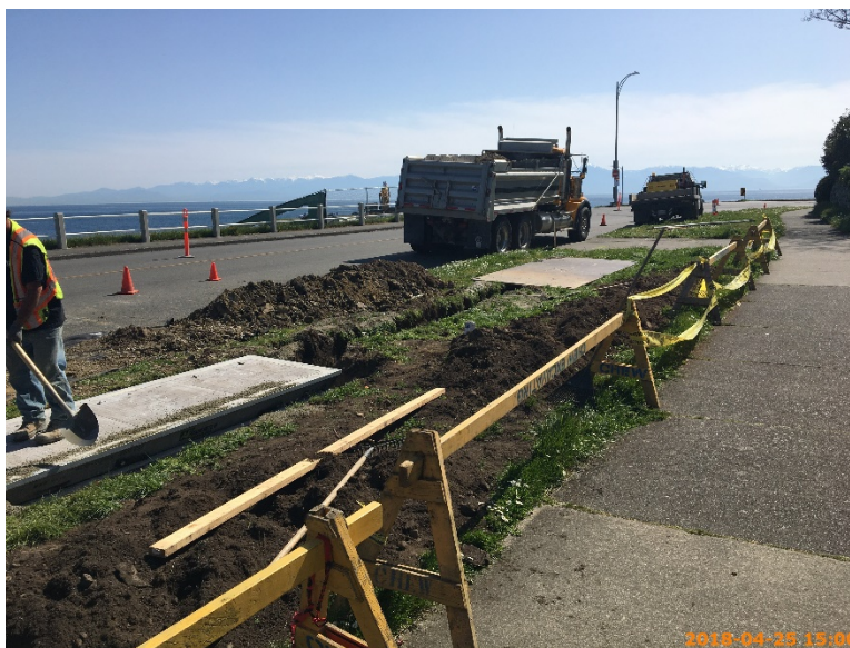
Figure 10 – BC Hydro contractor installing duct bank and pull box on north side of Dallas Road
