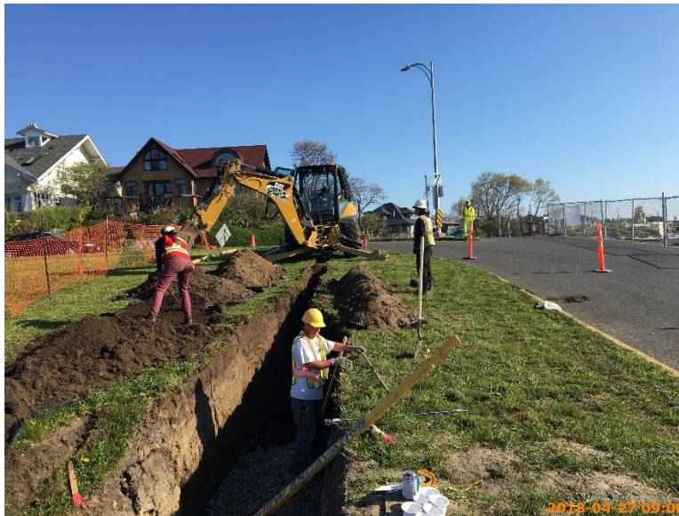
Figure 9 – BC Hydro contractor excavating for duct bank and pull box west side of Clover Point Road.
