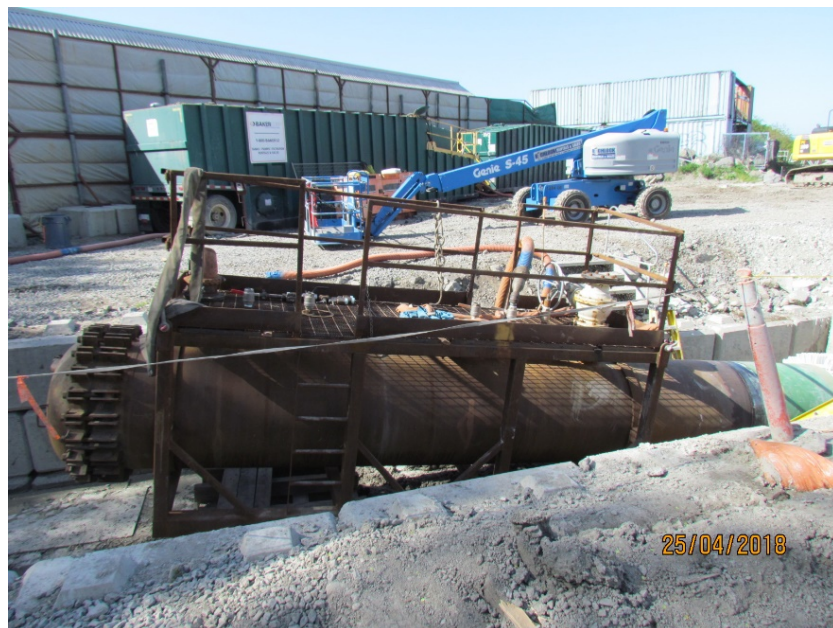
Figure 7 – Hydrostatic test head installed on the Ogden end of the Harbour Crossing pipe.
