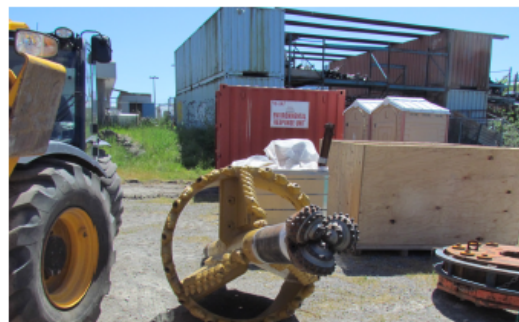
The horizontal directional drill bit being used to drill the hole for the cross-harbour undersea pipe that will go from Ogden Point to McLoughlin Point.
