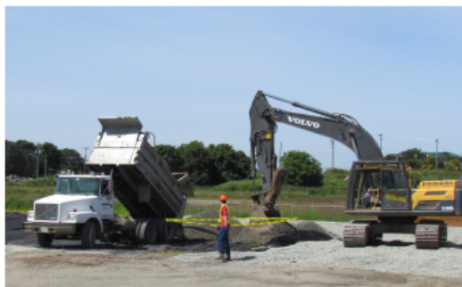
Crews placing aggregate in a laydown area for the McLoughlin Point Wastewater Treatment Plant in Esquimalt.
