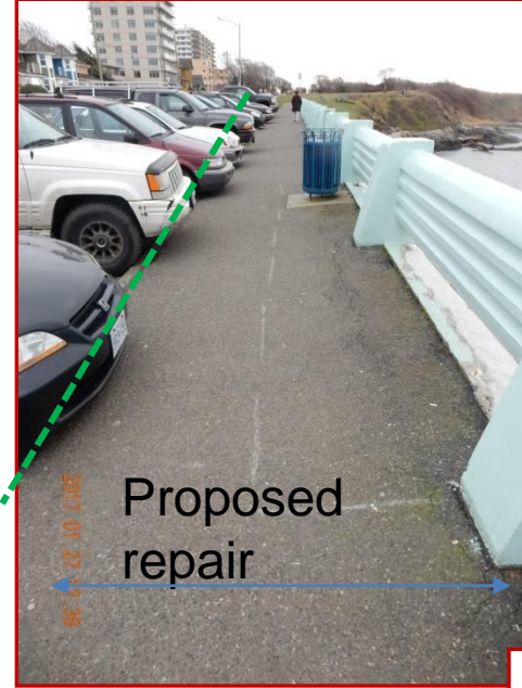
Subsidence Fractures due to undercutting
