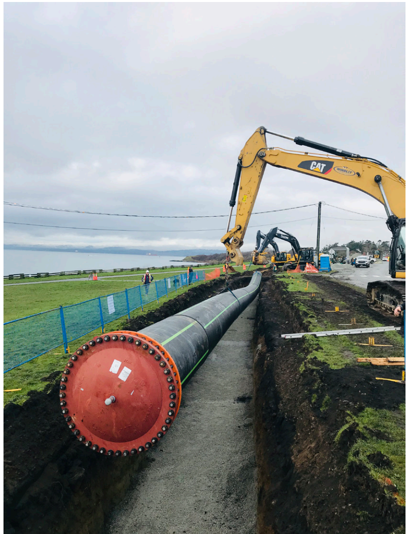
The 1.2m diameter Clover Forcemain is being lowered into the trench near Clover Point. There will be single lane alternating traffic on Dallas Road during construction.
