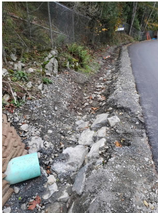
Photo 15: • Spill pathway after spill clean-up
