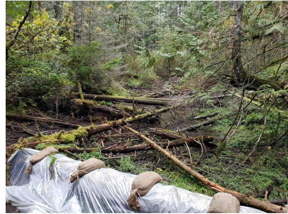
Photo 10 • Wetland after spill clean-up
