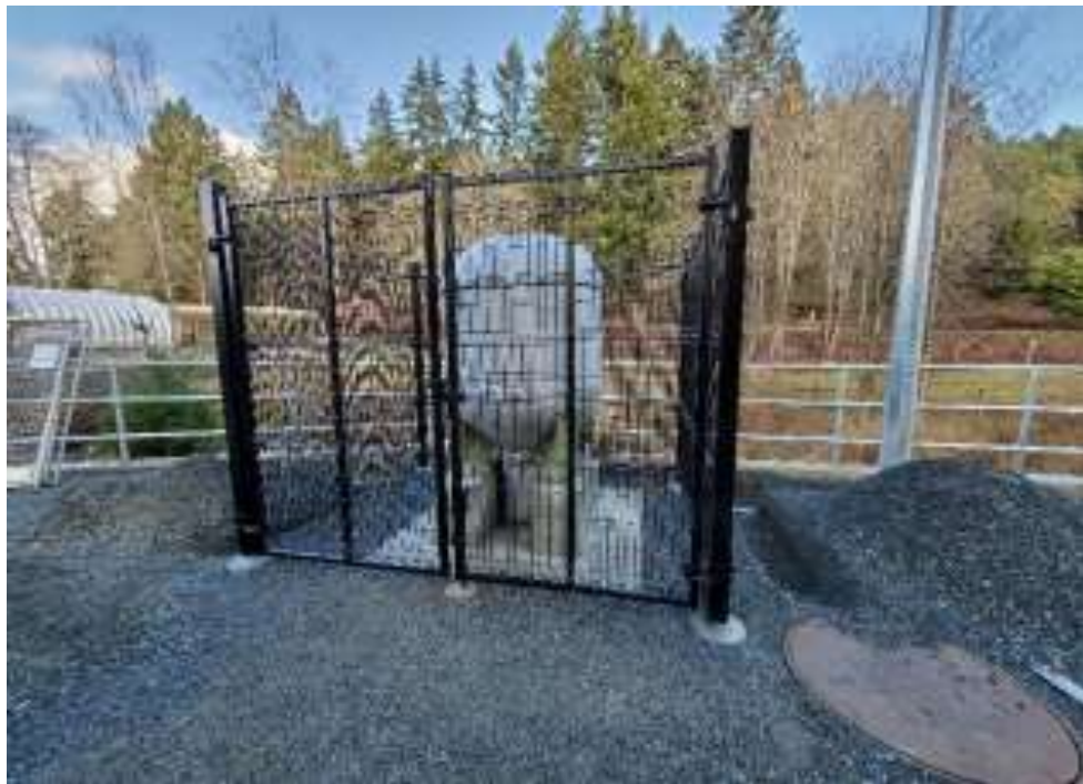
Figure 11–Residual Solids Pump Stations– Tower Fence installed around the Surge Tank
