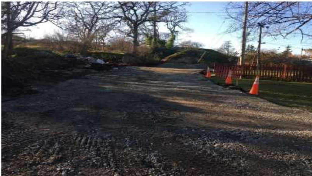
Figure 10–Residual Solids Pipes – View of site from Bewdley Ave facing south
