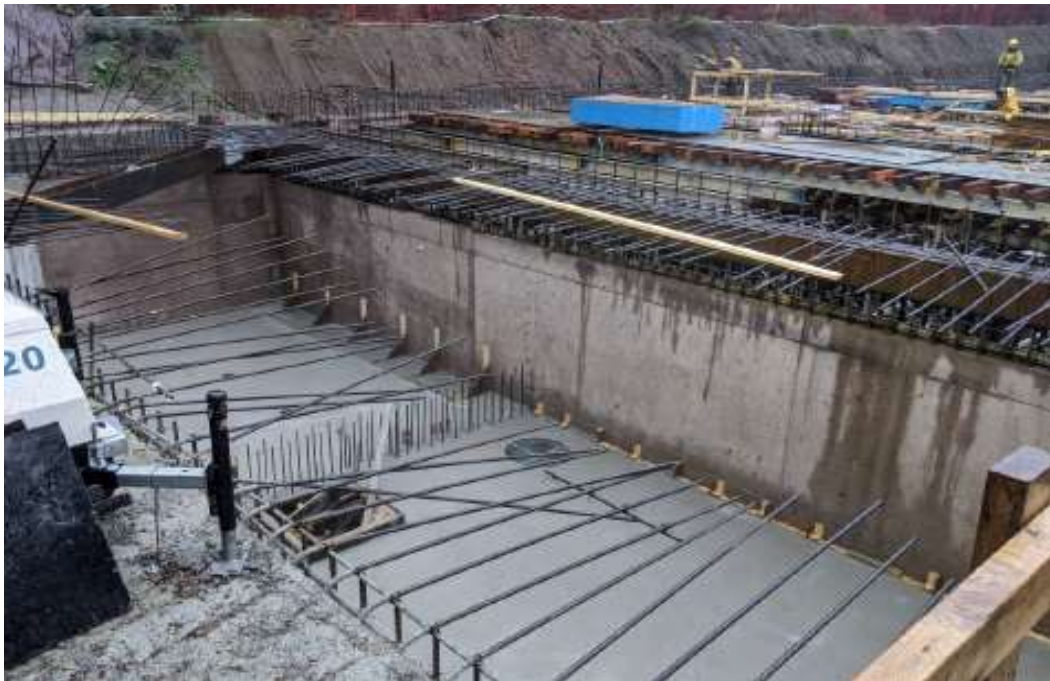
Figure 14–Arbutus Attenuation Tank- Concrete Pour completed at the South end of the tank
