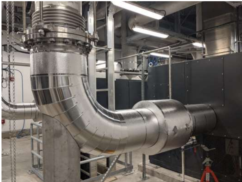
Figure 2– McLoughlin Point Wastewater Treatment Plant- Blower outlet process air piping insulation installed.
