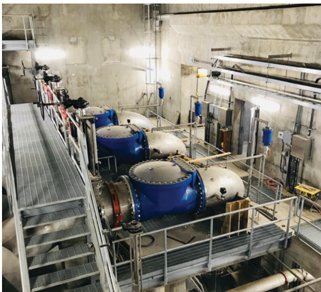
New pumps at the Clover Point Pump Station.
