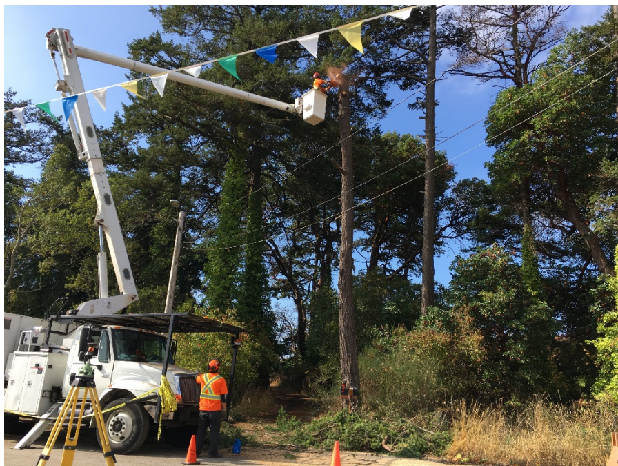
Figure 8 - Arborist cutting around power lines
