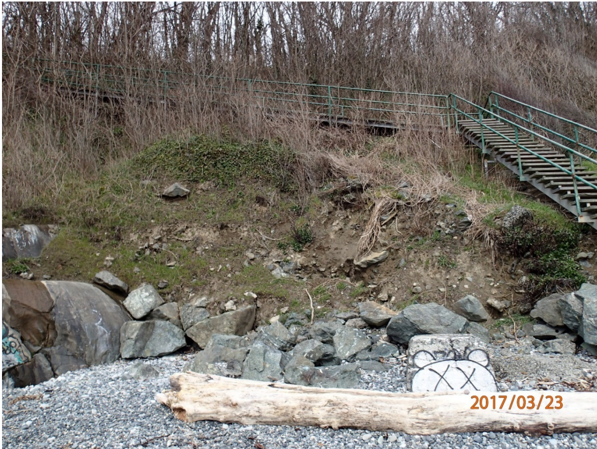
Figure 7 Suspected fill material below Douglas Street stairwell exposed by wave erosion.
