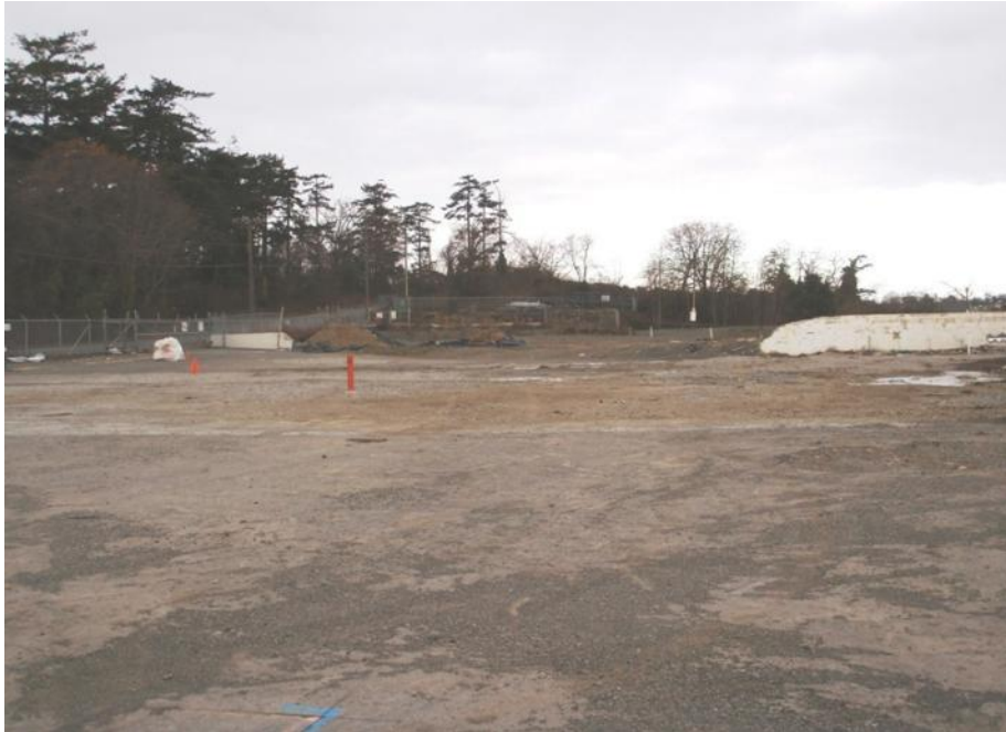
Figure 5-19. McLoughlin Point property, looking north. Asphalt pad and concrete slab capping in foreground.
