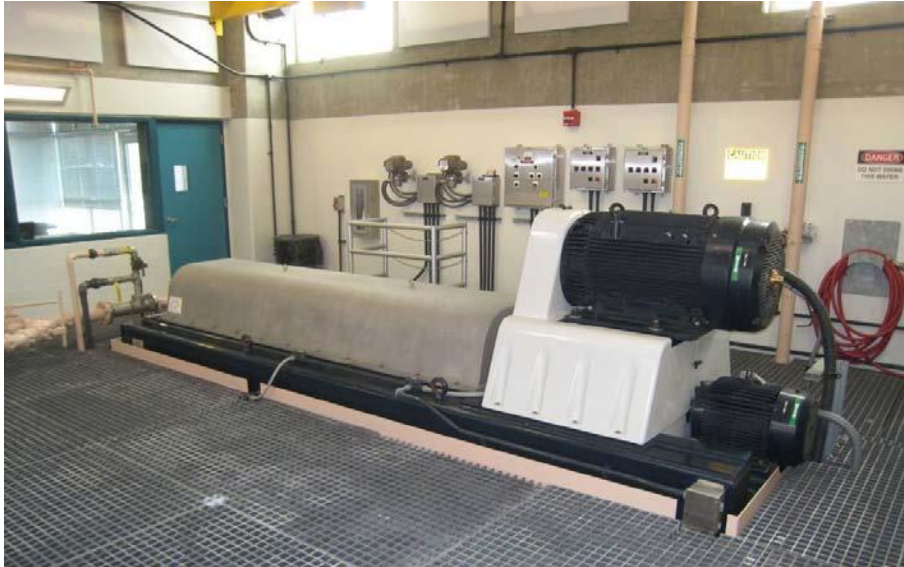
Figure 5.4 – High-speed Centrifuge: South Treatment Plant, Renton, Washington
