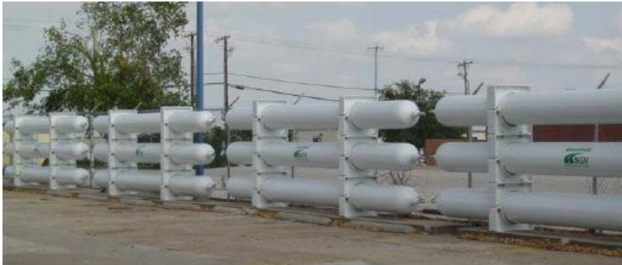
Figure 6.6 – Compressed Gas Storage Cylinders
