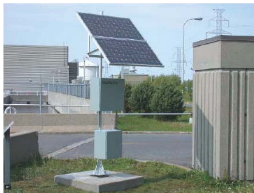
OdoWatch™ E-Nose at Water Treatment Plant
