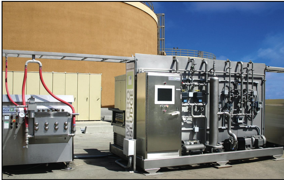
◀ The MicroSludge System at the JWPCP plant in LA County, one of the largest wastewater treatment plants in North America.
