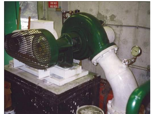
A typical small-scale PAT installation. Source: Associated Engineering
