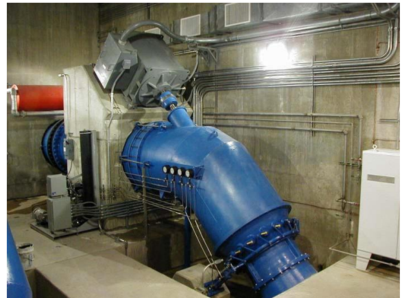
A 300 kW axial turbine installation.
