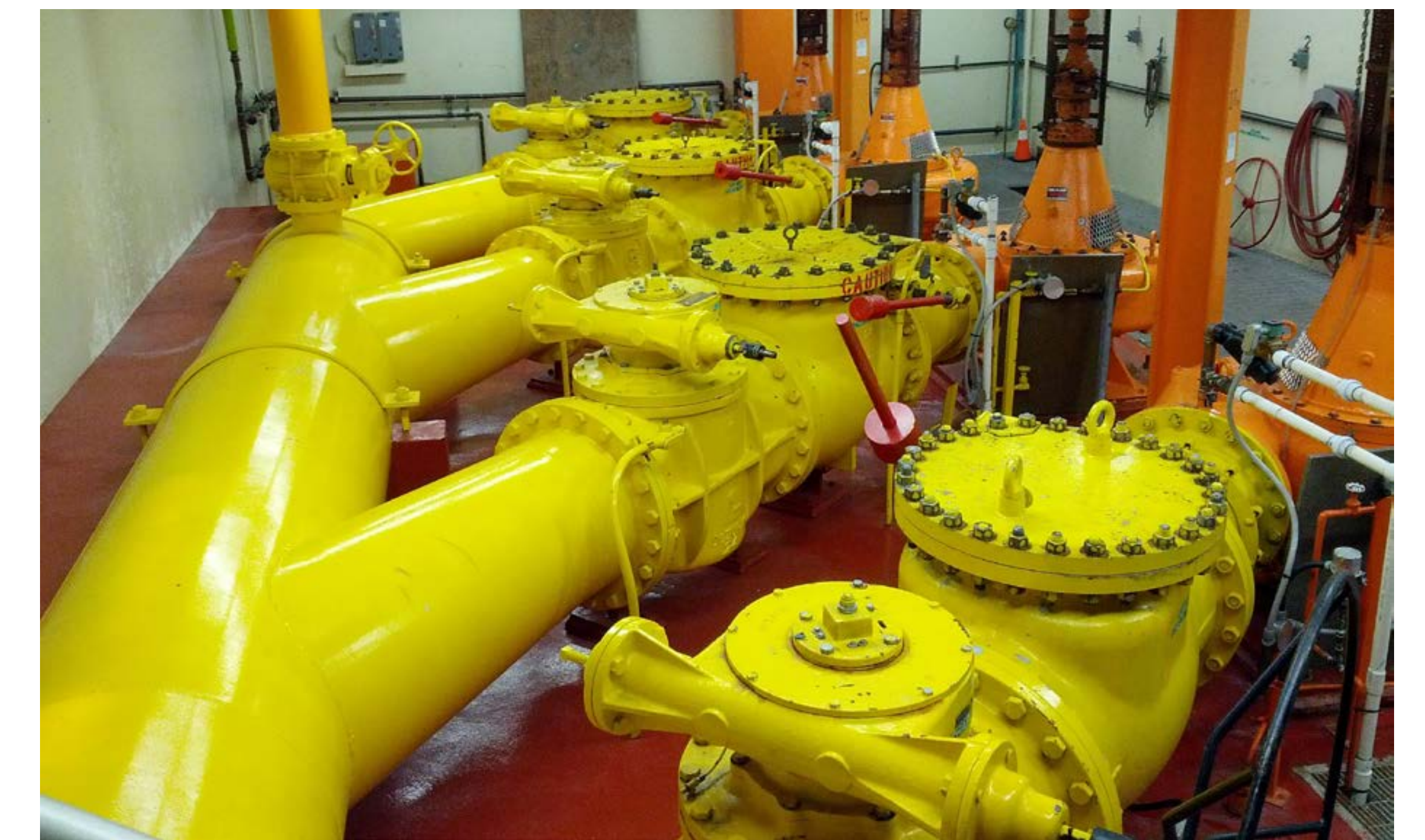
>> Pumps at Clover Point Station
