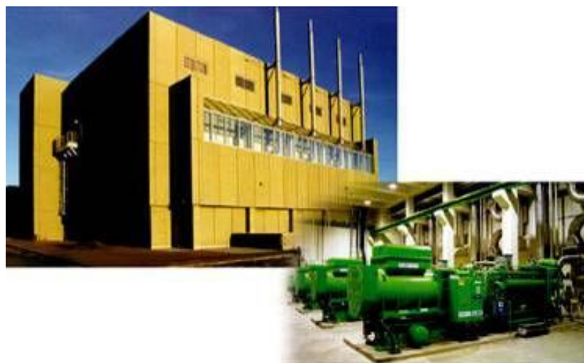
Figure 6.2 – 4-MW Cogeneration System at Metro Vancouver’s Annacis Island WWTP
