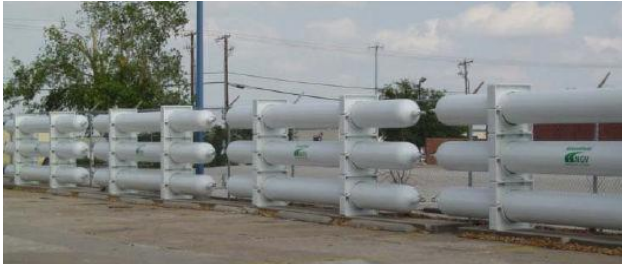
Figure 6.6 – Compressed Gas Storage Cylinders
