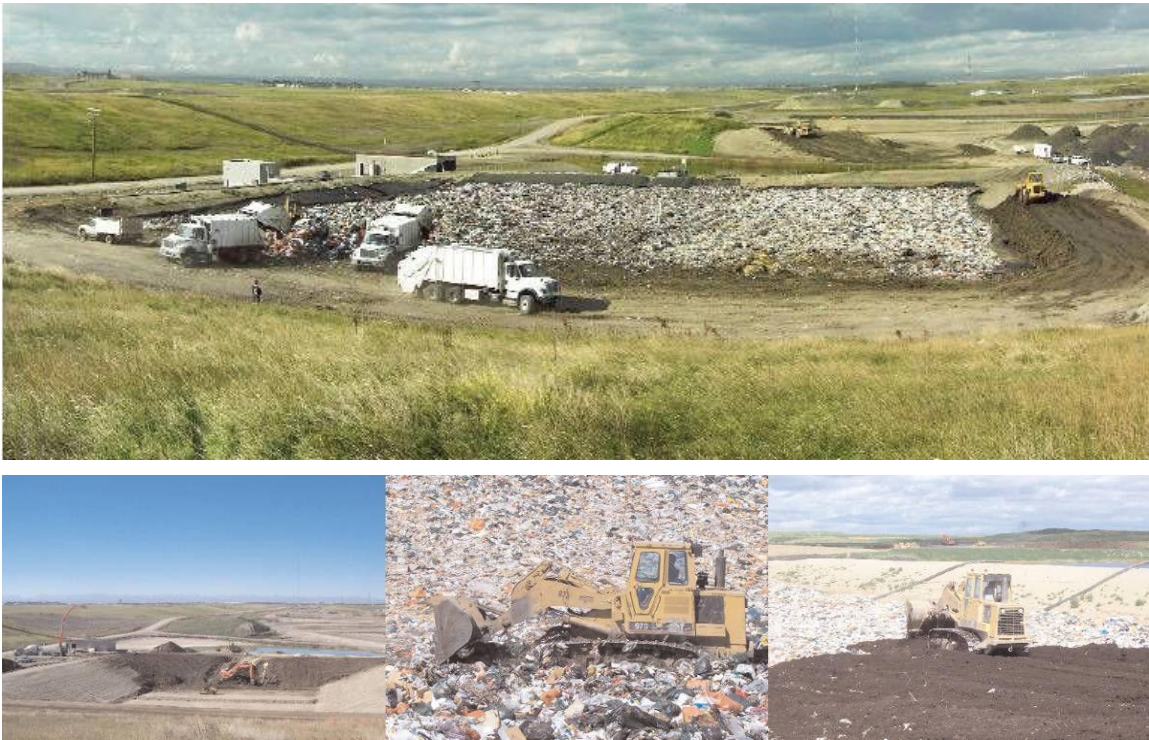
Figure 3.13 – Biocell in Operation (Stantec, 2006)
