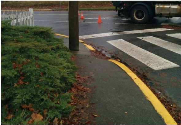
▲ A hydro pole obstructing a sidewalk and crosswalk on Cadboro Bay Rd.
