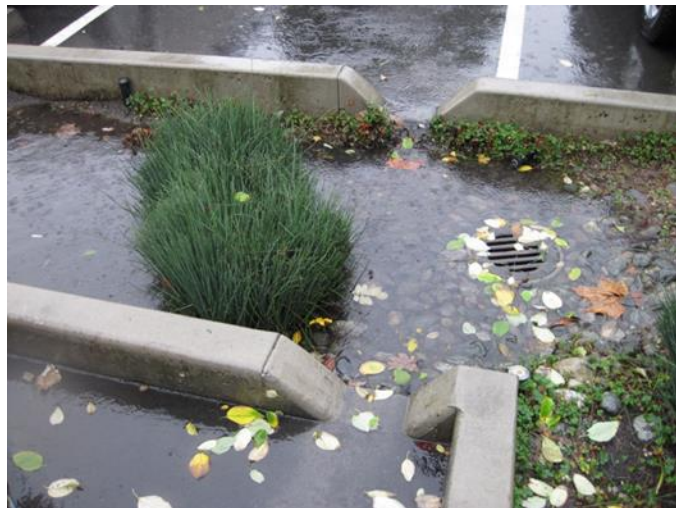
Figure 2 Flat drains such as in the infiltration planter can easily get clogged with leaves
