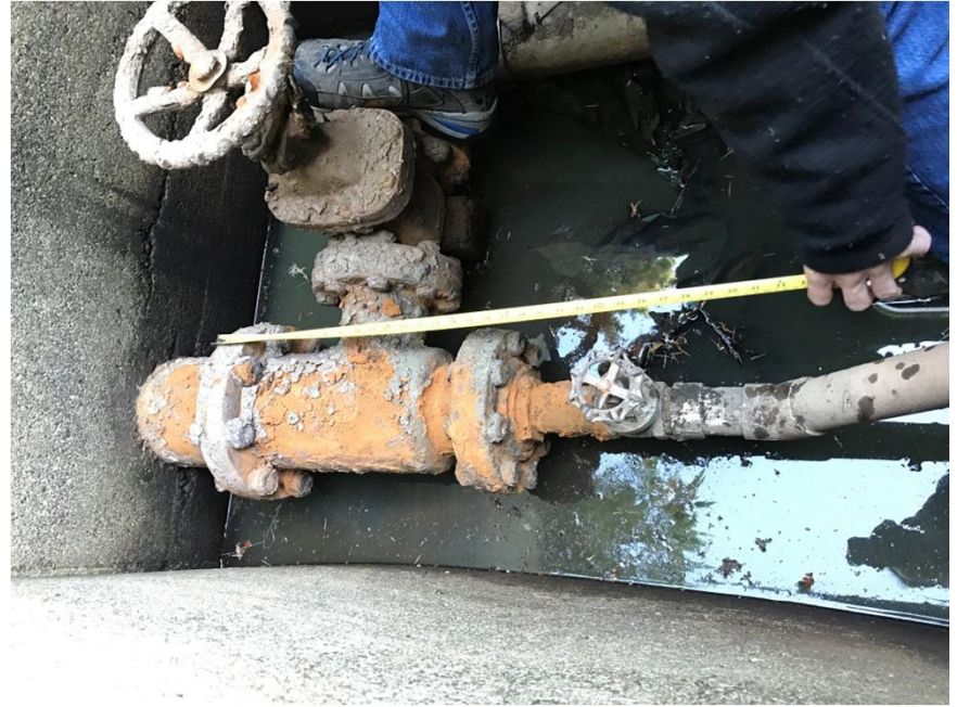
Photograph #2 – Top View: Low Level Outlet Chamber Infrastructure Deposit build-up partially removed
