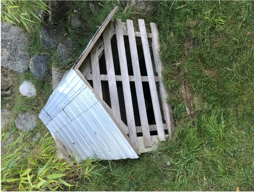
Photograph #1: Low Level Outlet Chamber and Housing Located on downstream face of Gardom Pond Dam
