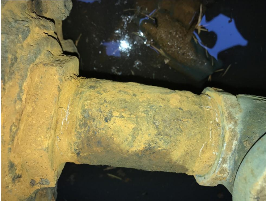
Photograph #7 – Top view: 50 mm dia. Irrigation Feed Deposits and scaling removed Note presences of pipe threads and Teflon tape
