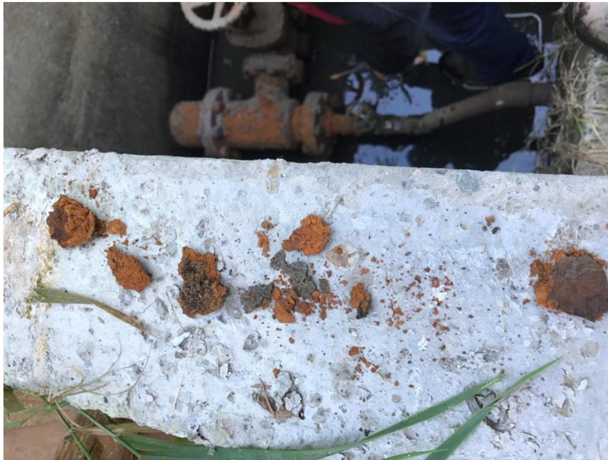
Photograph #3: Deposit Build-Up Typical samples collected from top of fittings & piping
