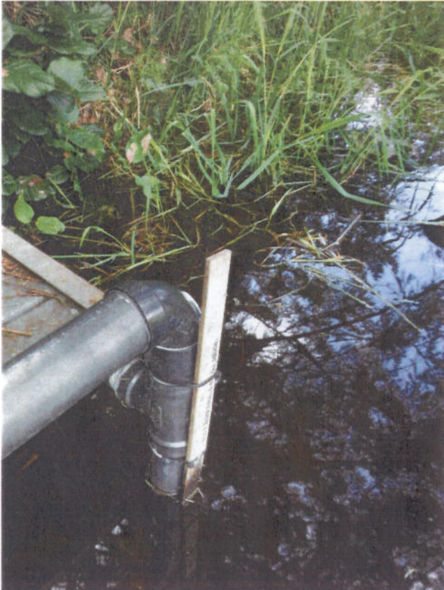
Gardom Pond Reservoir Water Level Gauge
