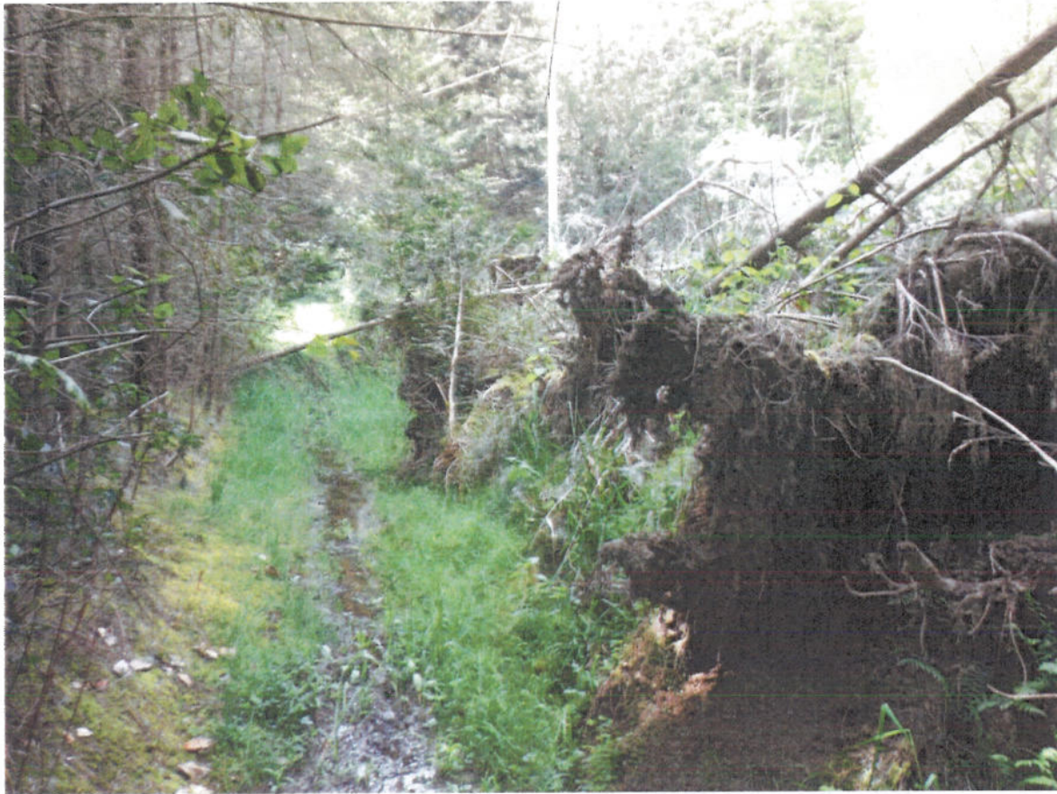
Gardom Pond Spillway Channel – Damaged channel sidewalls require remediation.
