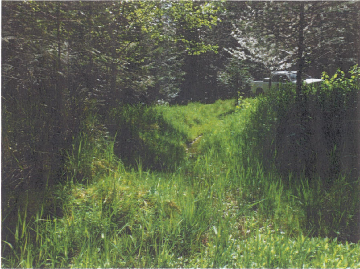
Gardom Pond Spillway Channel – Routine brushing in channel leading up to road culvert required.
