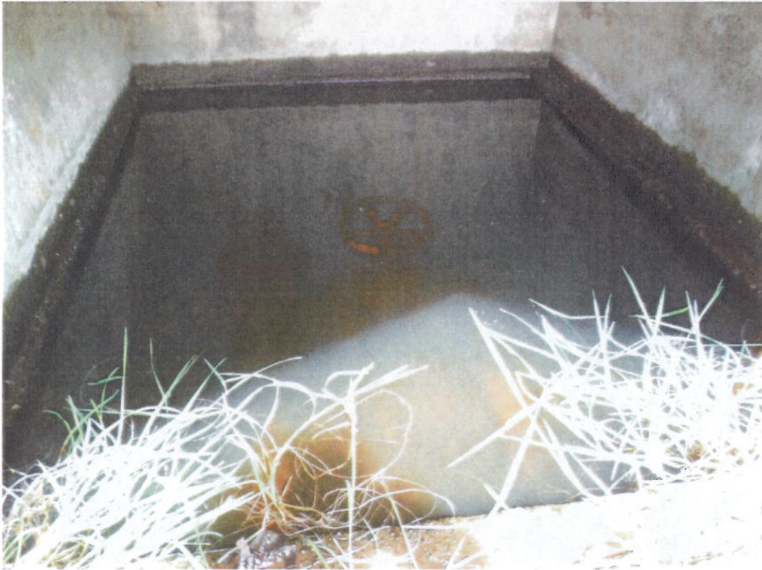
Gardom Pond Dam valve chamber at downstream toe. Water level staff gauge should be installed. Drain pipe should be installed to keep chamber dry and to monitor seepage into the chamber.
