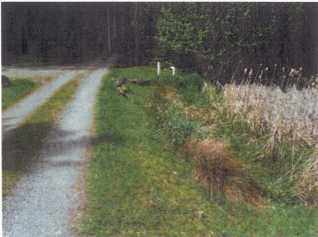
Gardom Pond Dam – Ruts in the road on the dam crest should be filled. Upstream face should be brushed to facilitate inspection.
