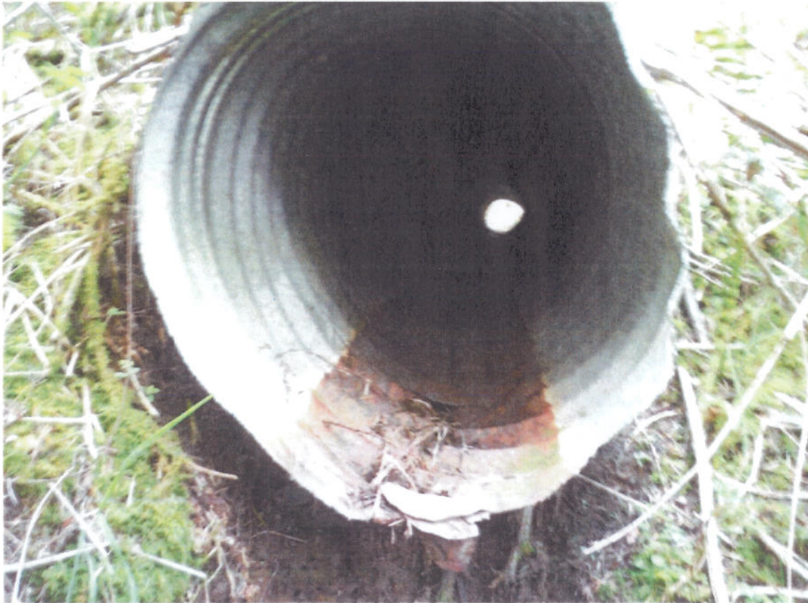
Gardom Lane Spillway Culvert – Road culvert should be replaced.
