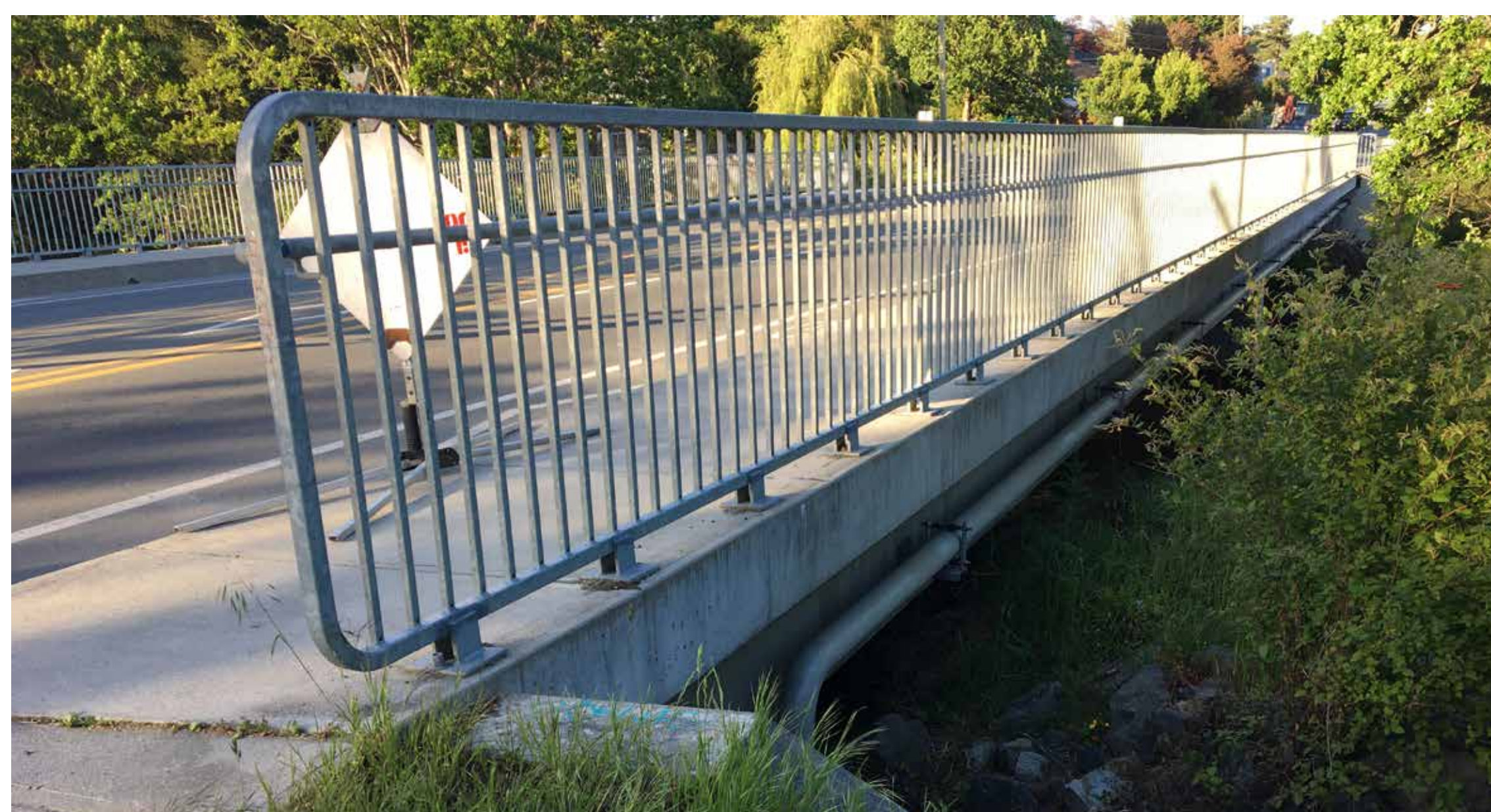
Conveyance pipe on bridge
