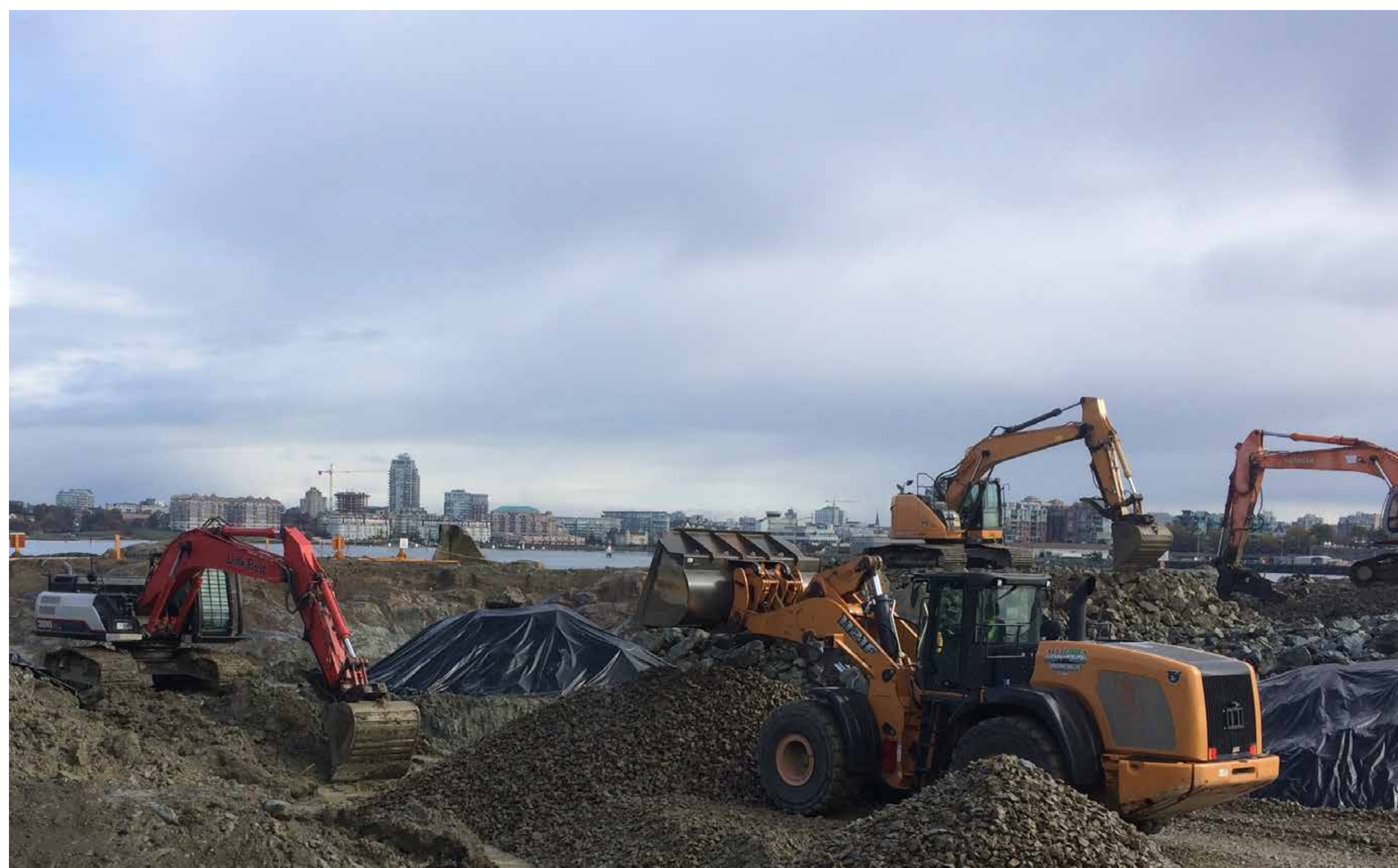
Construction is underway at the McLoughlin Point Wastewater Treatment Plant in Esquimalt
