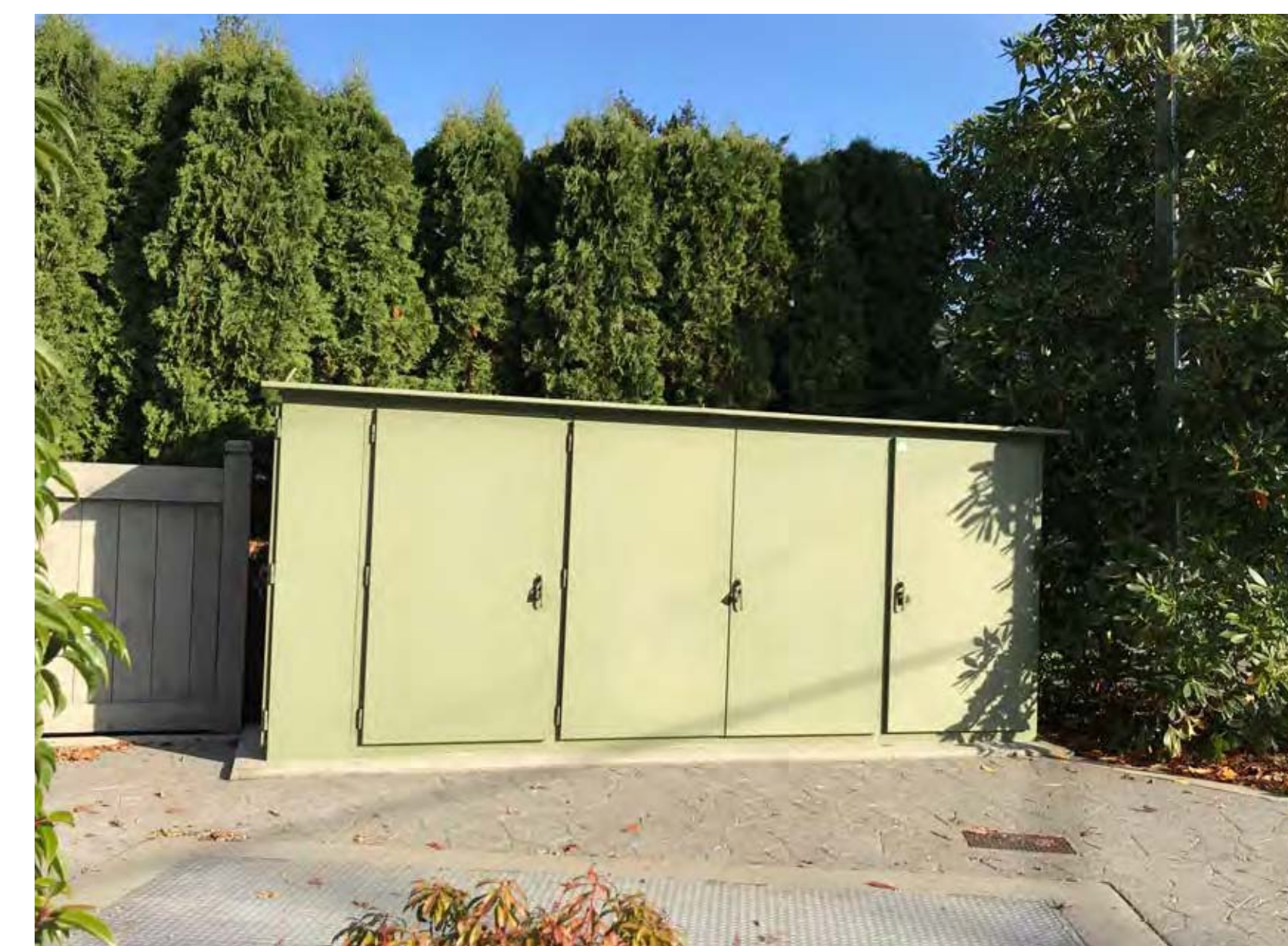
Vantreight Pump Station, Saanich
