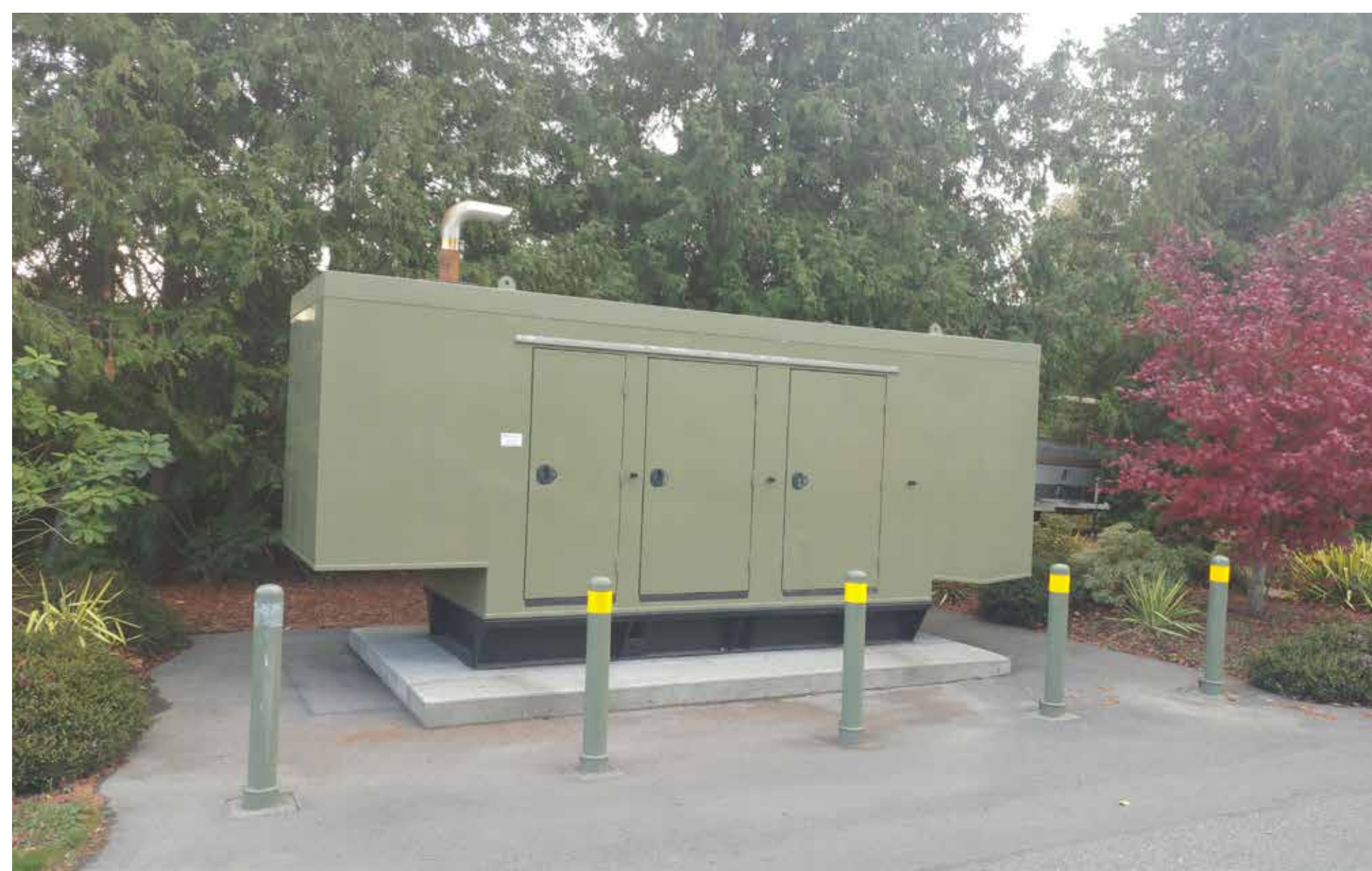
Albina Street Pump Station, Saanich
