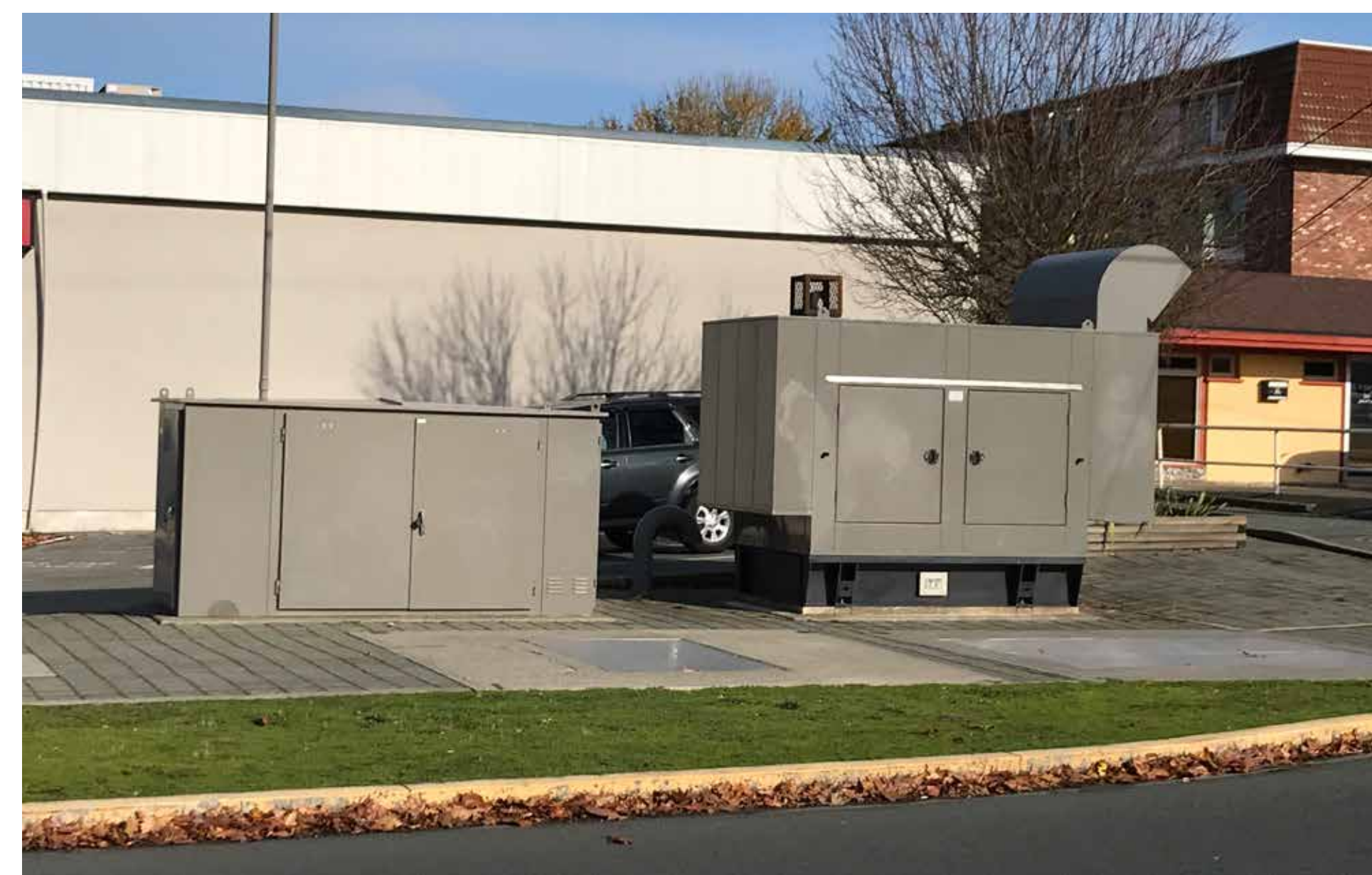
Pear Street Pump Station, Saanich
