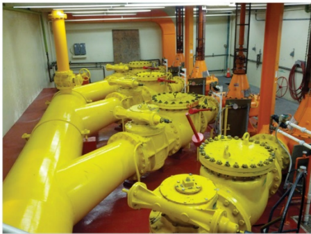
Clover Point Pump Station – Inside
