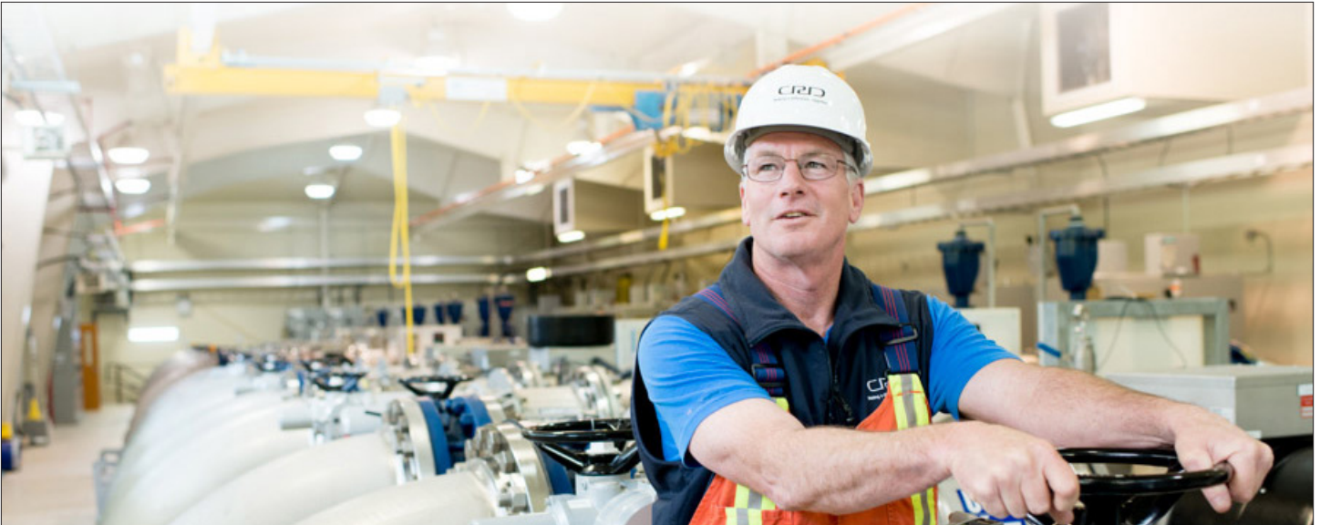
Japan Gulch Ultraviolet Disinfection Plant
