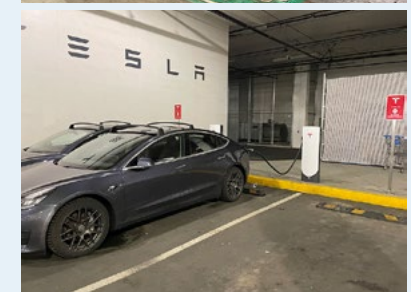
Examples of underground parking with EV charging (Centennial Square Parkade [top] and Tesla Supercharging hub at Uptown Mall [bottom])
