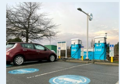
Examples of parking lots shared by several businesses with EV charging (Anytime Fitness at 5120 Cadboro Bay Road [top] and Saanich Plaza [bottom])
